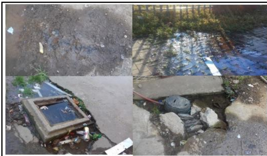
Figure 8.14 – Street/Town Leakages in Alice Community
