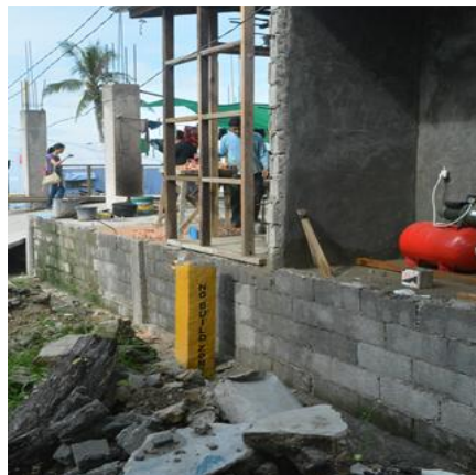
A part of the building of the showroom was already within the no build zone issued by the government after Typhoon Yolanda.
