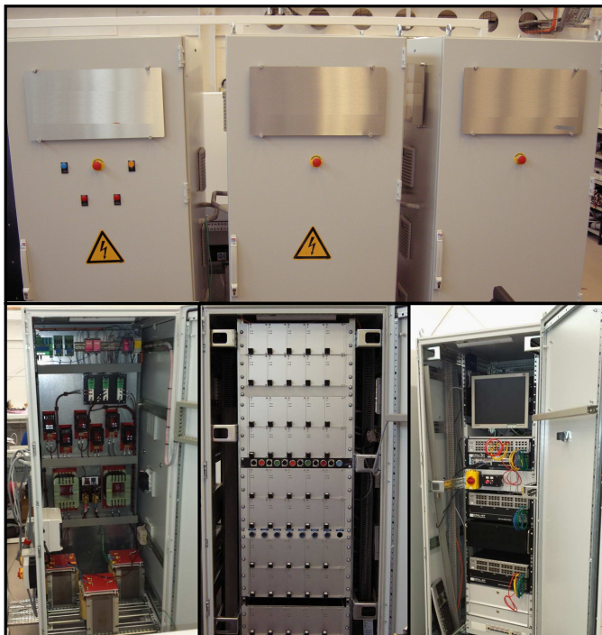
Fig. 30. Cabinets for components interfacing SMs with AC and DC sides (left), SMs (middle), and control hardware (right)
