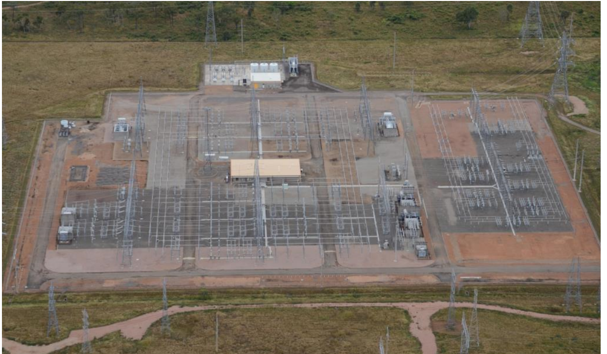
Figure 1.1: Typical view of a electrical substation. Earth grid is typically installed half a meter below the earth's surface all around the substation.
