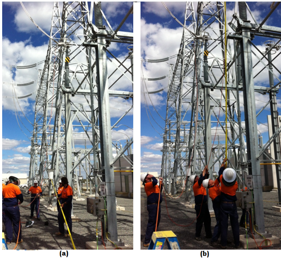
Figure 2.10: (a) Transmission grid isolator opened (b) Generator fed into the transmission line
