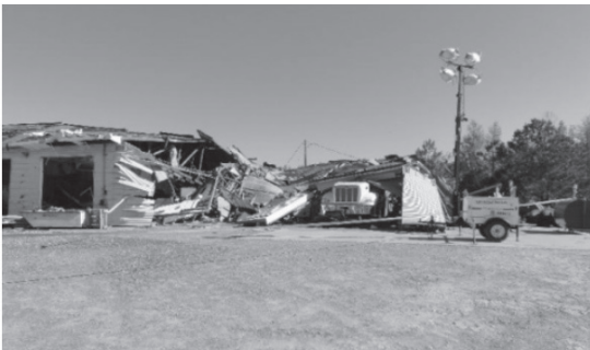
Figure 7 Damaged tanker and garage at Surry Power Station (source: NOAA.gov), available at: http://www.erh.noaa.gov/akq/wx_events/severe/apr_16_2011/Surry2.JPG
