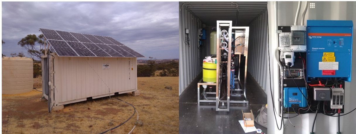
Figure 8: Muresk PVRO Unit, Exterior (left), RO Unit (middle), Power Board (right)
