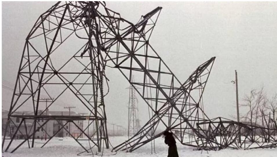
Figure 1-1: Woman walking by a collapsed transmission pylon causing massive power outage in Quebec (Robert Galbraith/Canadian Press).
