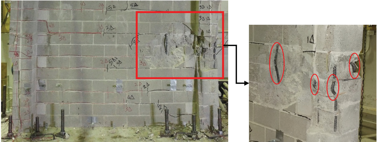
Figure A.6 Final damage state and failure of wall W7
