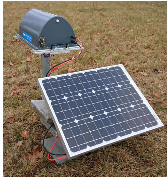
Fig. 2: ECR112 installation with solar panel power supply.
