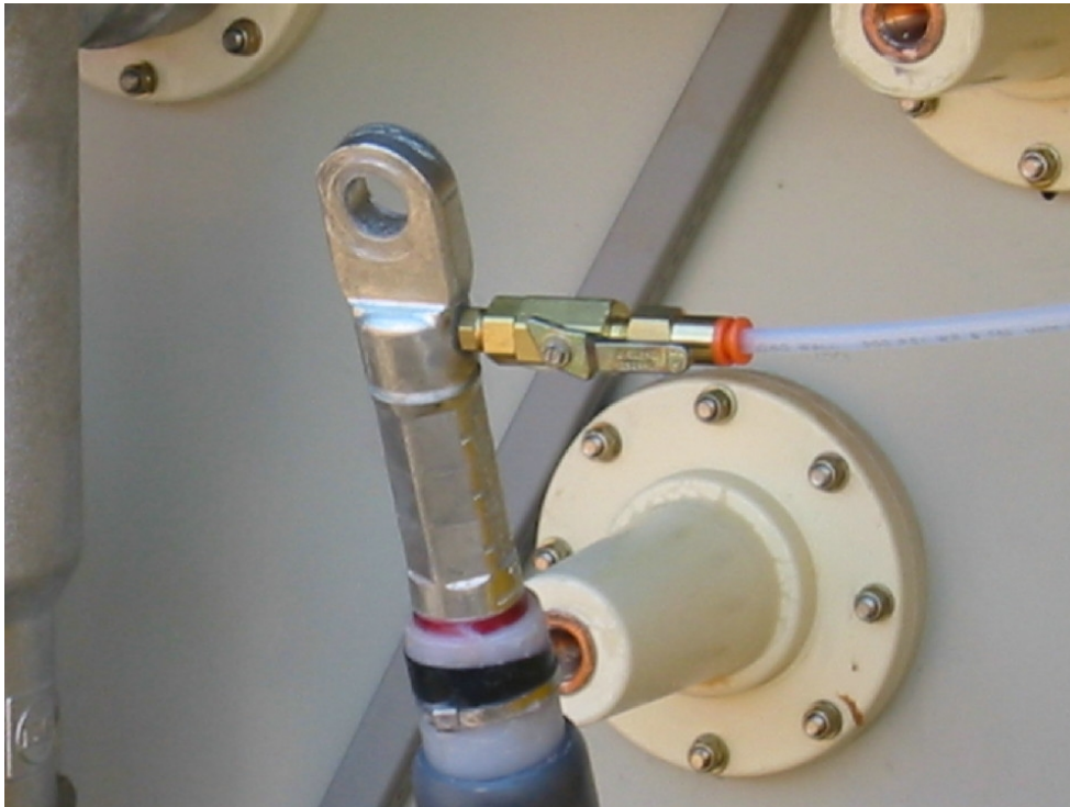
Figure 3.3: Image of a CableCure termination, showing the port (connected to the hose) into which the fluid is pumped into the cable.
