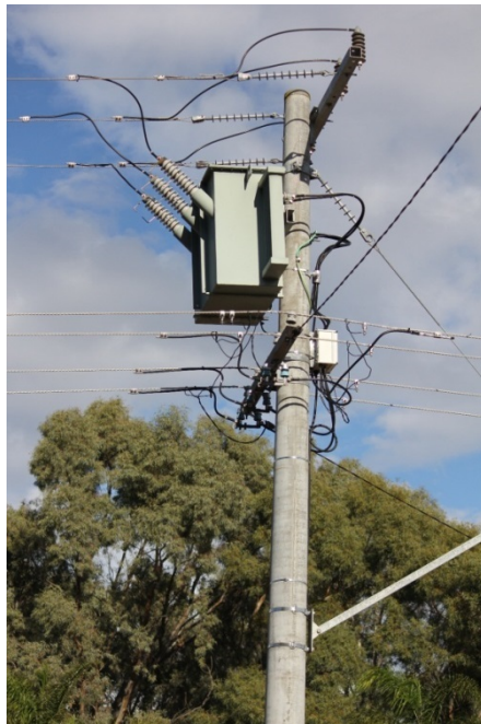
Figure 3-3. Pole-mounted transformer and data logger under study (Pavetta TX1)
