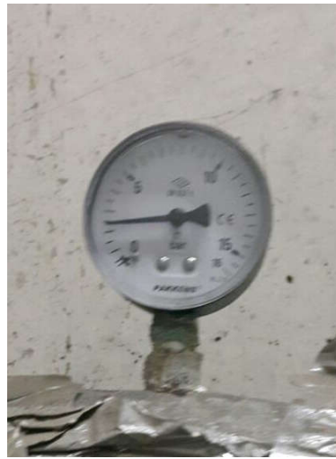
Figure 6-48 Pressure gauge for Pump 2
