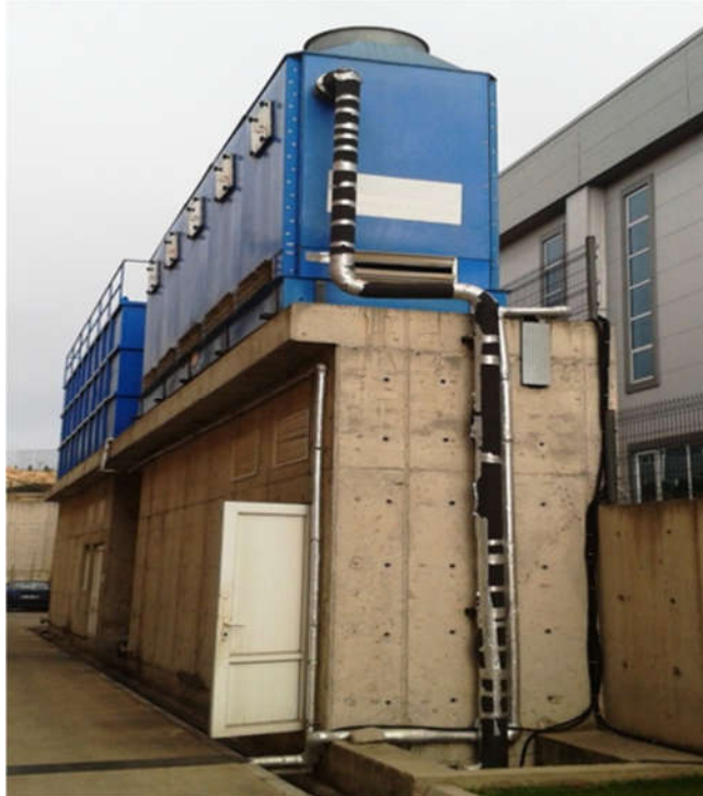
Figure 6-46: Cooling Tower used for sand reclamation system and quenching pool in the subject plant
