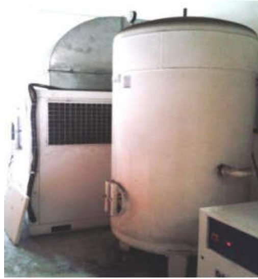
Figure G-3: Compressed air storage tank in the subject plant
