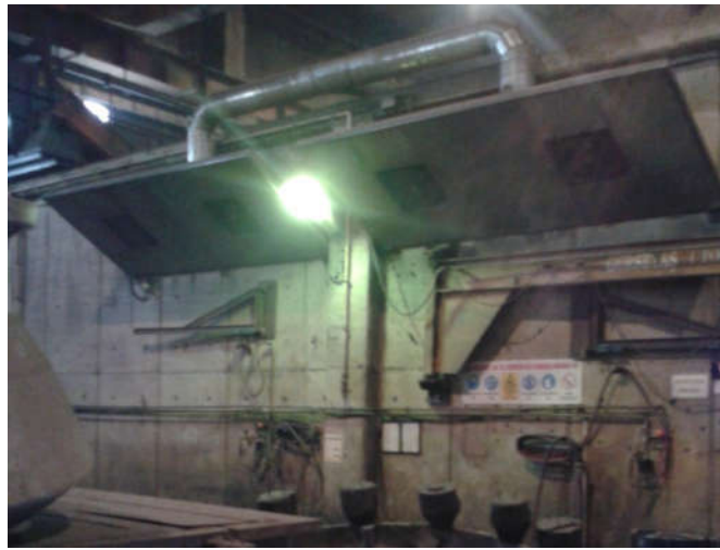
Figure 6-1 An example of local exhaust ventilation at one of the grinding stations in the subject plant (Photo taken by the Author)
