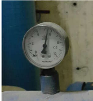
Figure 6-37: Pressure gauge of Pump 2 showing the total discharge head in bar
