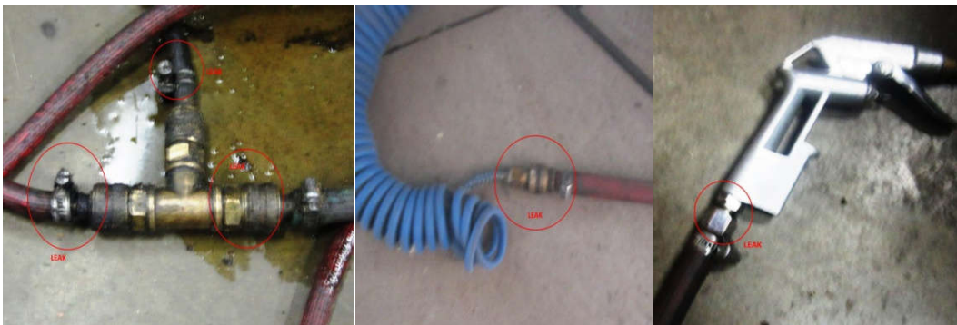
Figure 6-28: Most common areas which have air leaks in the subject plant compressed air system
