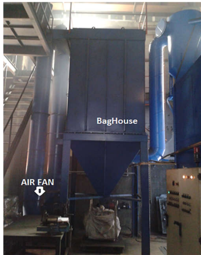
Figure G-8: Dust collection unit of the abrasive blasting system
