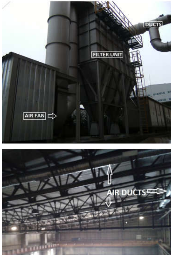
Figure 6-4: The ventilation system of the plant: air fan, filter unit, and ducting system
