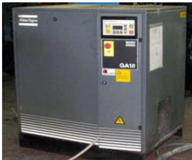
Figure G-2: Compressor 2 in the subject plant
