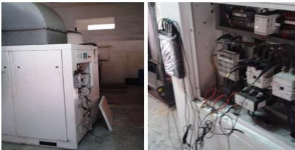
Figure G-1: Compressor 1 and power measurement of it in the subject plant
