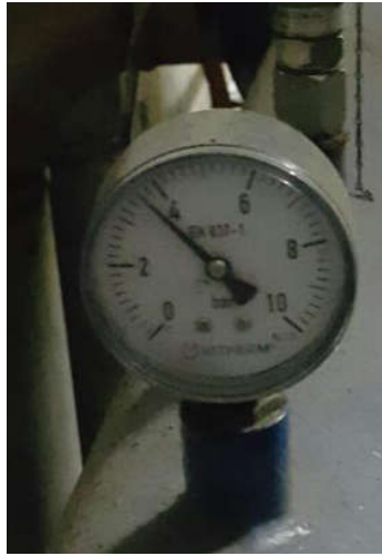
Figure 6-43: Pressure gauge for Pump 1 showing the discharge head in bar
