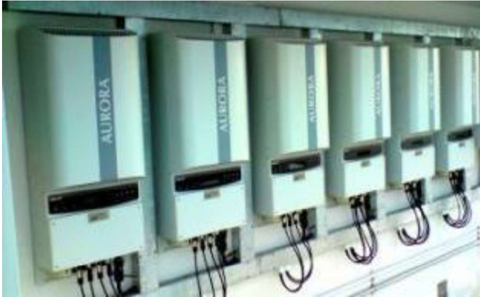
FIGURE A.4 INVERTERS USED IN THE PV SYSTEM
