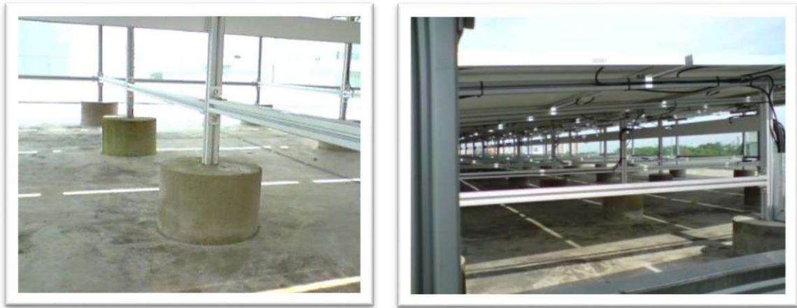
(a) Cement studs to hold panels down (b) Arrays are installed at 5^\circ inclination
