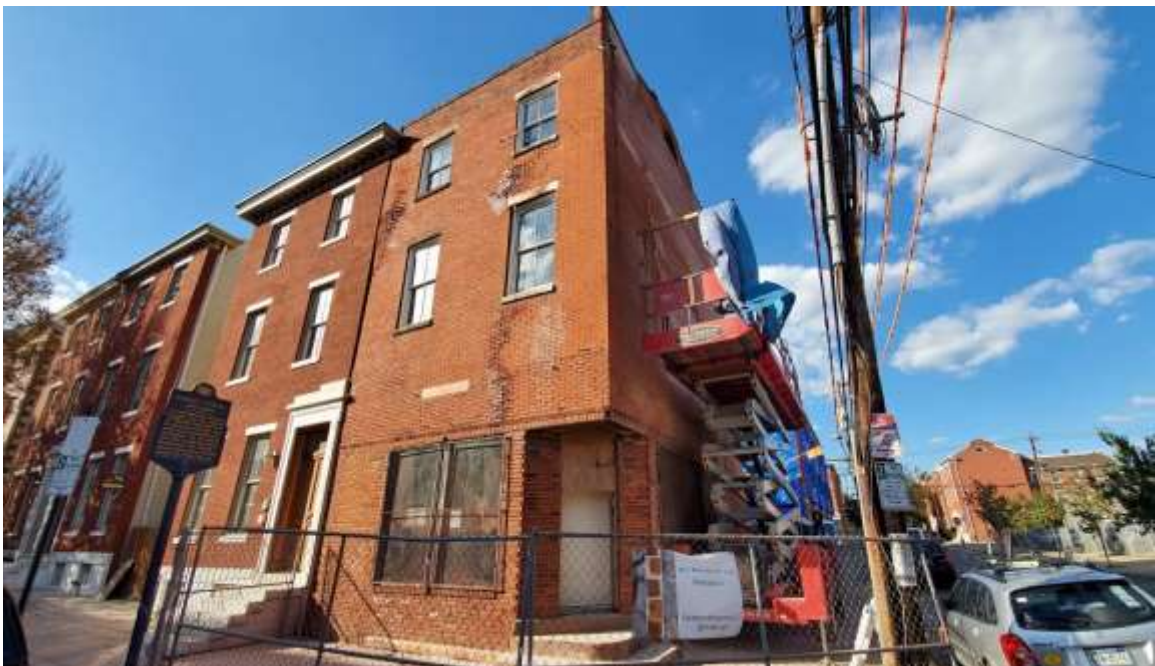
Figure 4.3. Work has recently begun to make repairs to the historic Robert Purvis House after it was placed into receivership. (Mark Henninger, Billy Penn, 2019)
