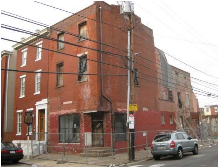
Figure 4.2. For years, the Robert Purvis House was left to deteriorate despite the efforts of the local community and other advocates. (OCF Realty, 2012)
