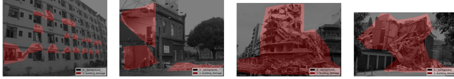
b (b) Annotated building-damage images
