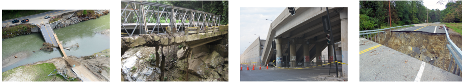
c (c) Original bridge-damage images
