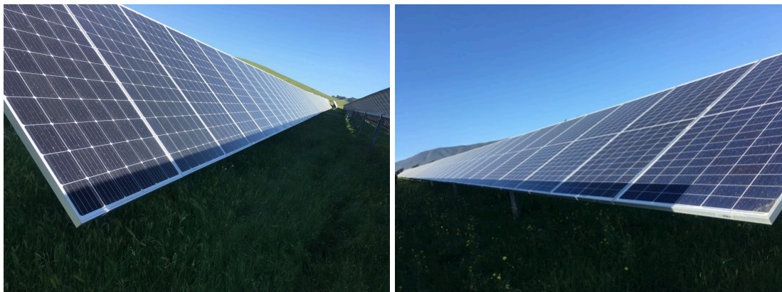
Figure 5.5: Inter-row Shading on Solar Panels Connected to Inverter 55 facing North (left) and Inverter 25 facing South (right) taken on 4/23/20
