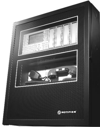
Figure 10. Notifier NFS-60 Fire Alarm Control Panel.
