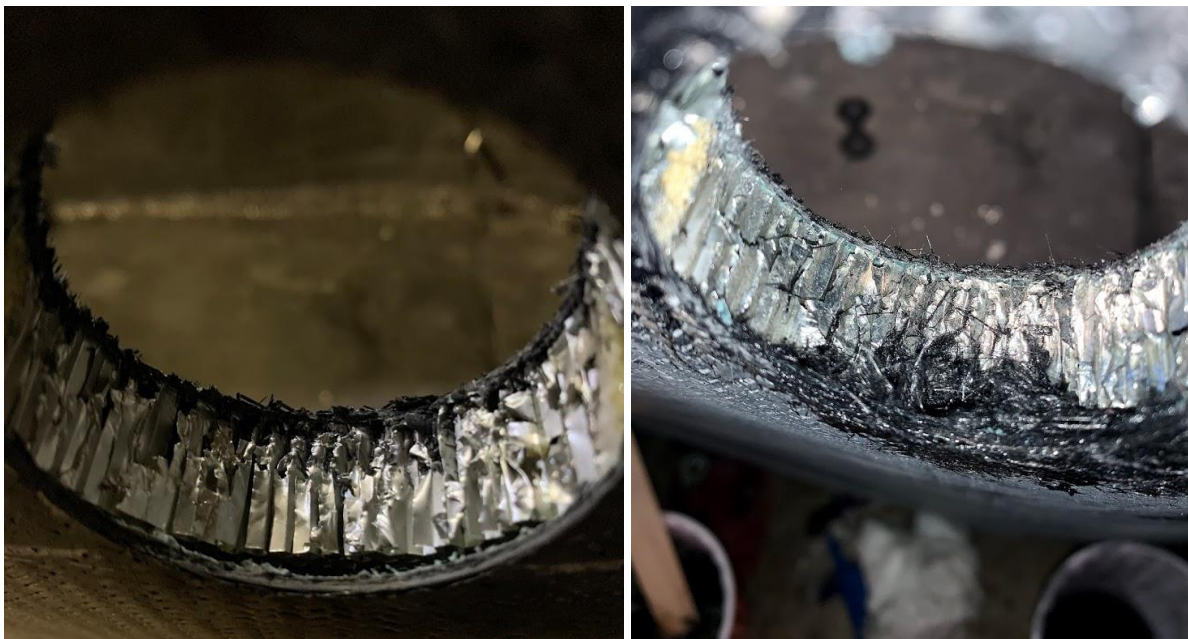
Figure 174. Delamination between core and outer skin (left) and a portion of subsequent repair (right).
