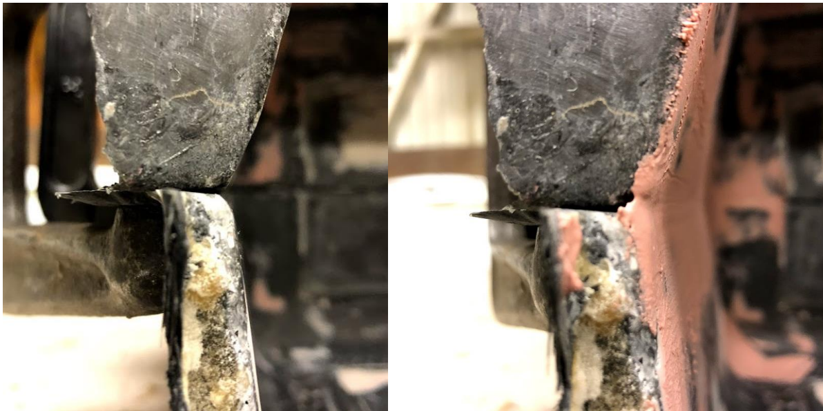
Figure 112. Seam gap shown on the left. Bondo body filler was used to fill the gap on the left.
