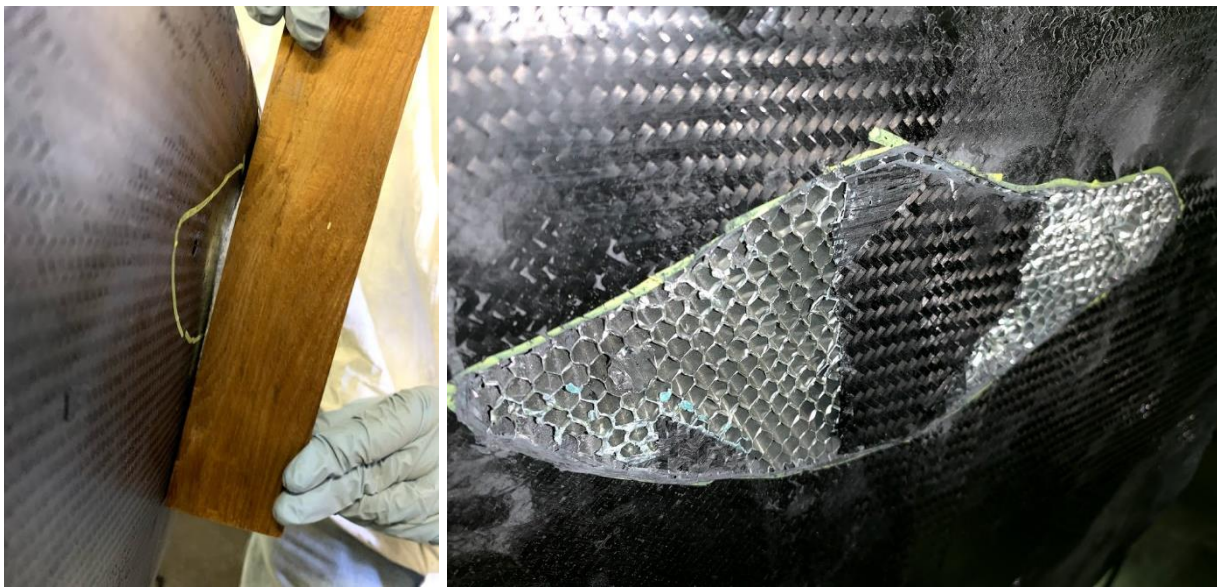
Figure 172. Dented chassis wall (left) and the outer skin removed (right) in order to perform a wet layup repair.
