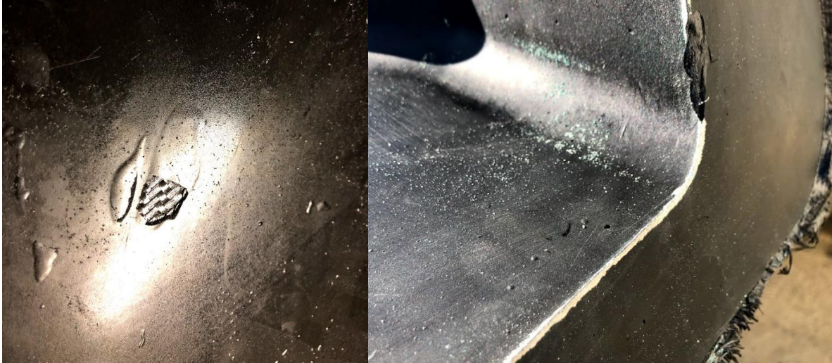
Figure 141. Voids in the surface coat crack along planar faces (left) as well as corners (right).
