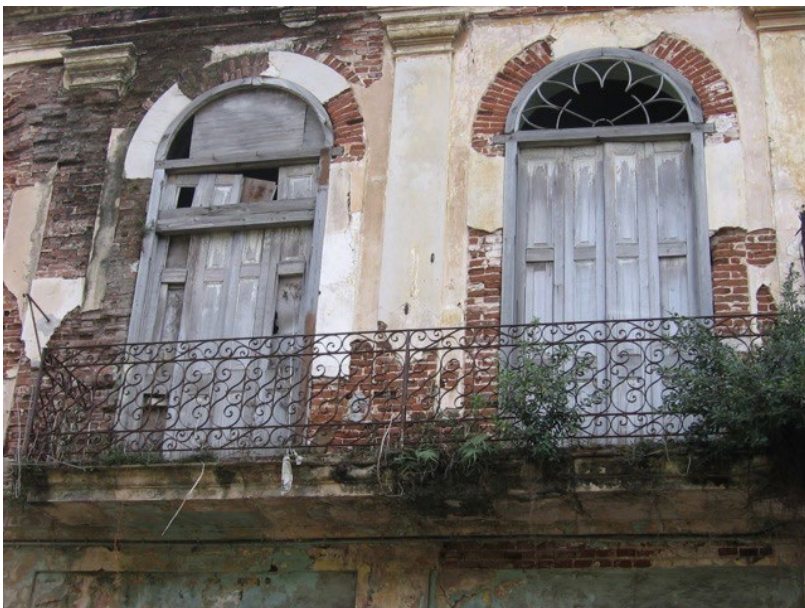
Cuba's government is renovating run-down buildings such as this one in the historic Havana Vieja.
