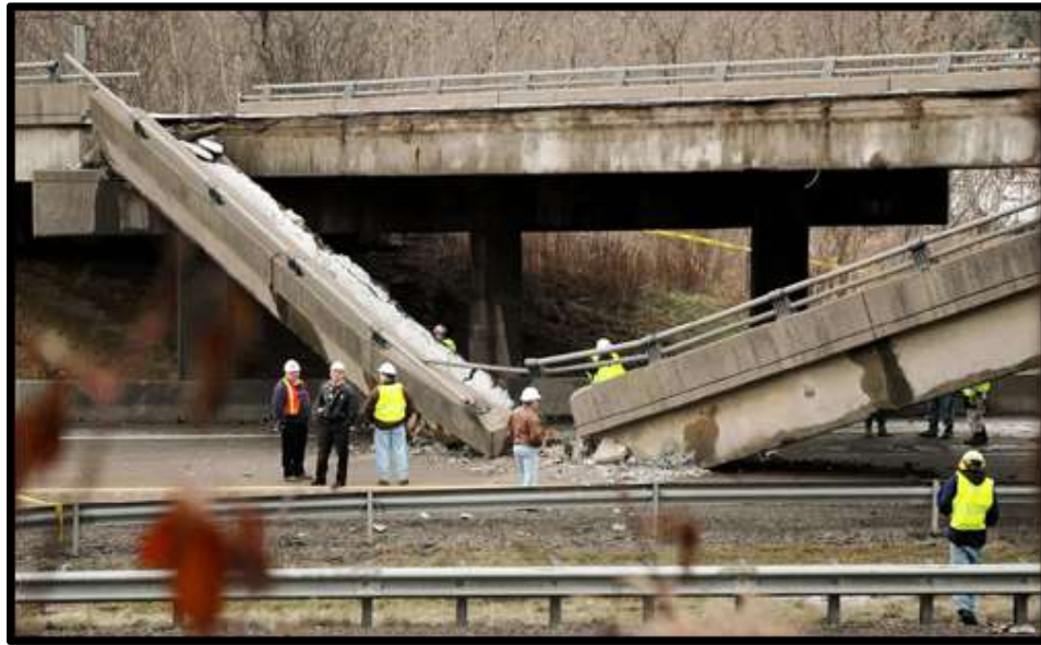
Figure 1.2 The Lake View Drive Bridge collapse (McCloskey, 2005).
