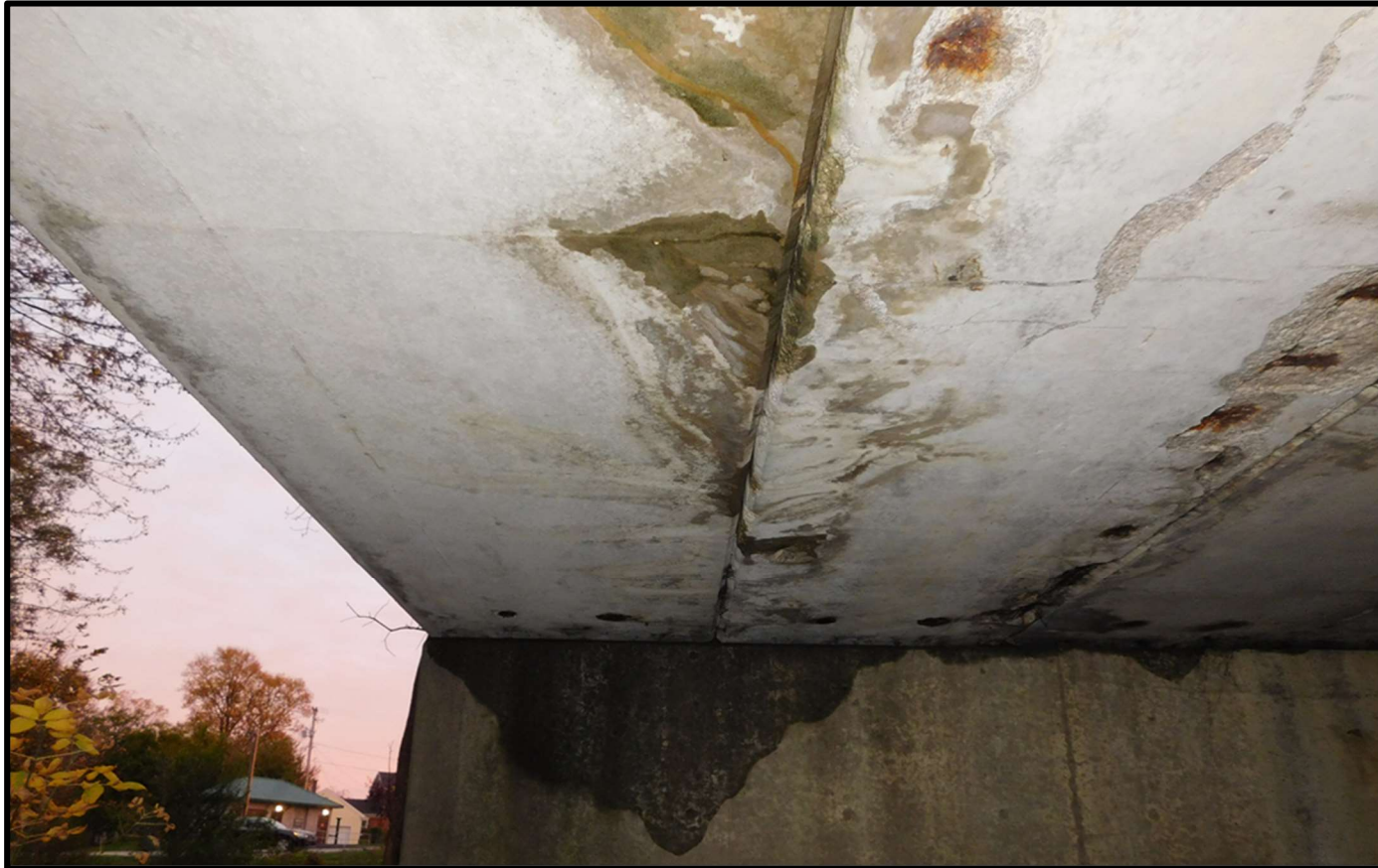
Figure 4.35 Water staining and efflorescence at the exterior longitudinal joint (Main Street).
