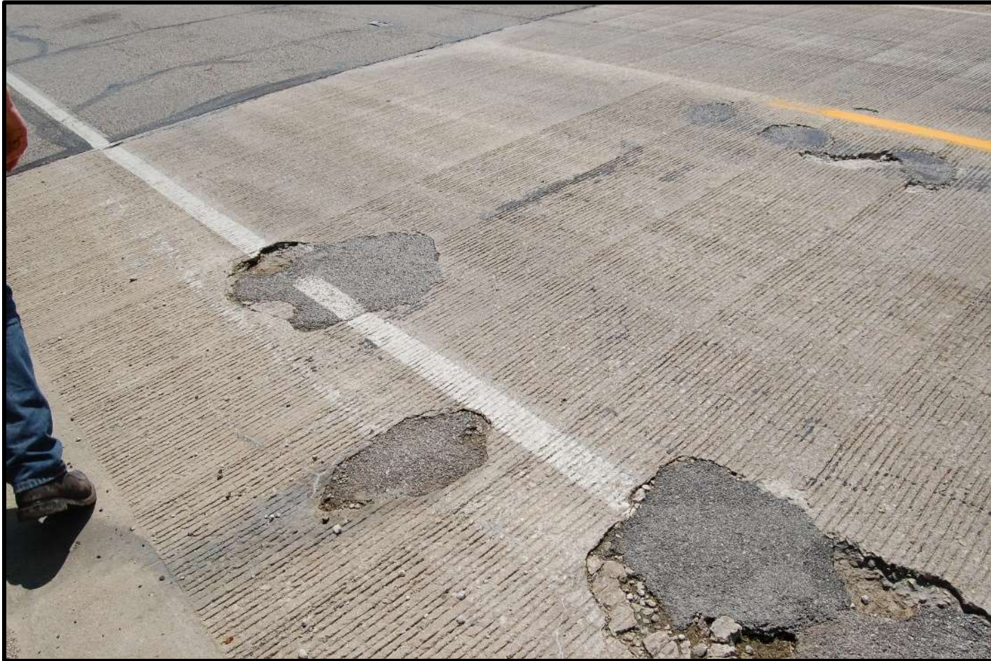
Figure 4.22 Potholes in wearing surface.
