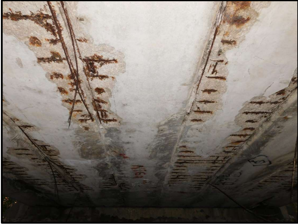
Figure 4.31 Spalling, corrosion, and fractured prestressed strand on west span.
