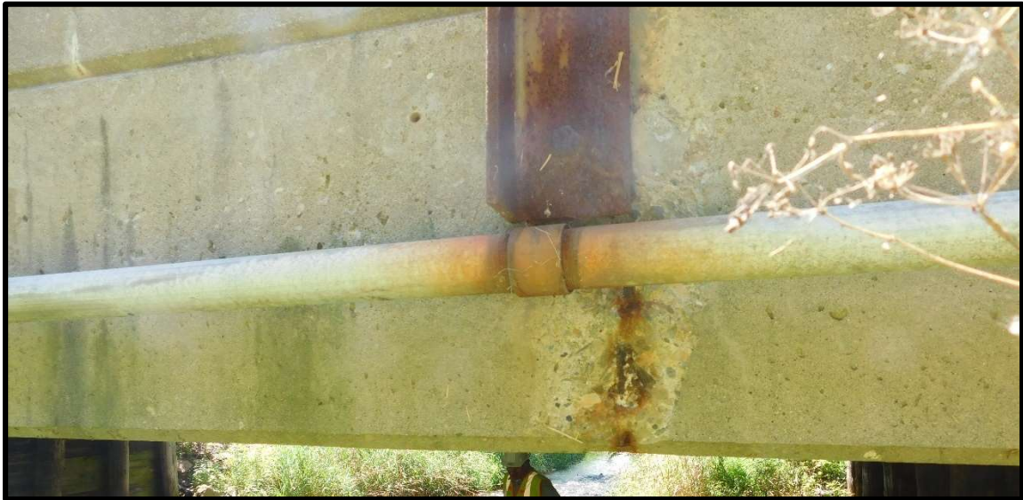
Figure 4.21 Spalling and exposed stirrup on the exterior face of Beam 8.
