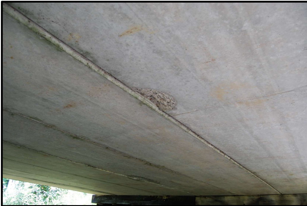
Figure 4.19 Spalling along bottom of longitudinal joint.
