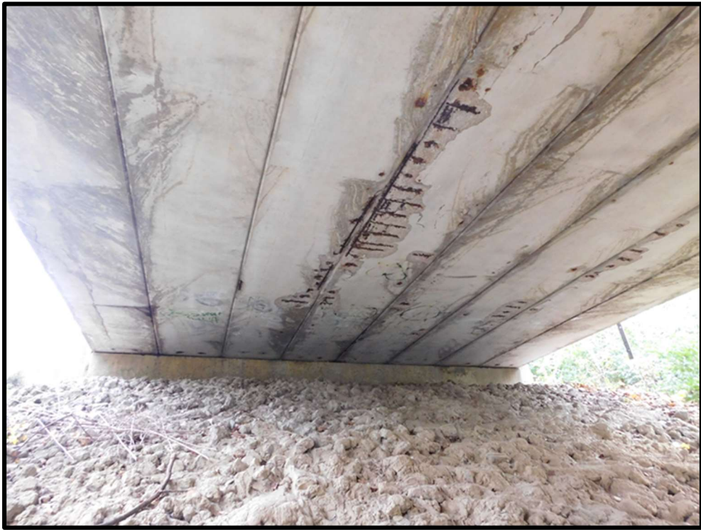
Figure 4.40 Corrosion of shear reinforcement (Main Street).
