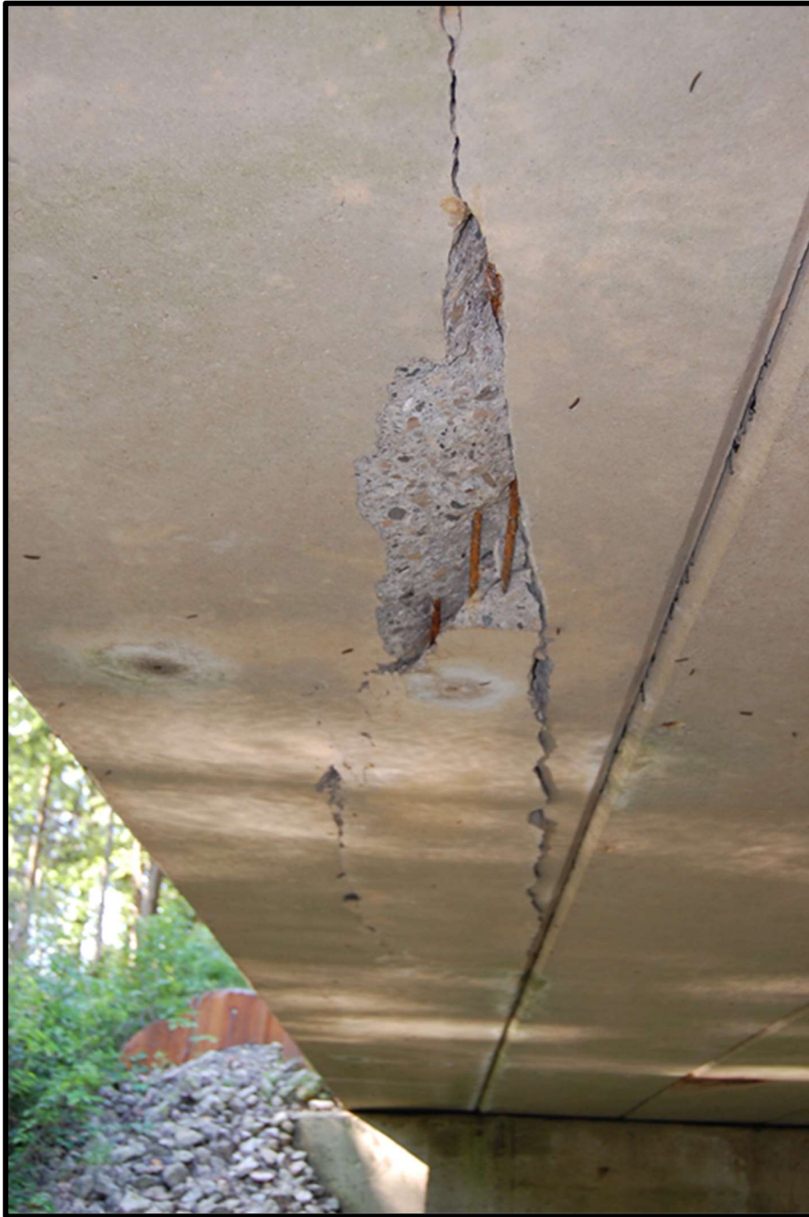
Figure 4.39 Spalling and exposed strands (Yellow Creek).
