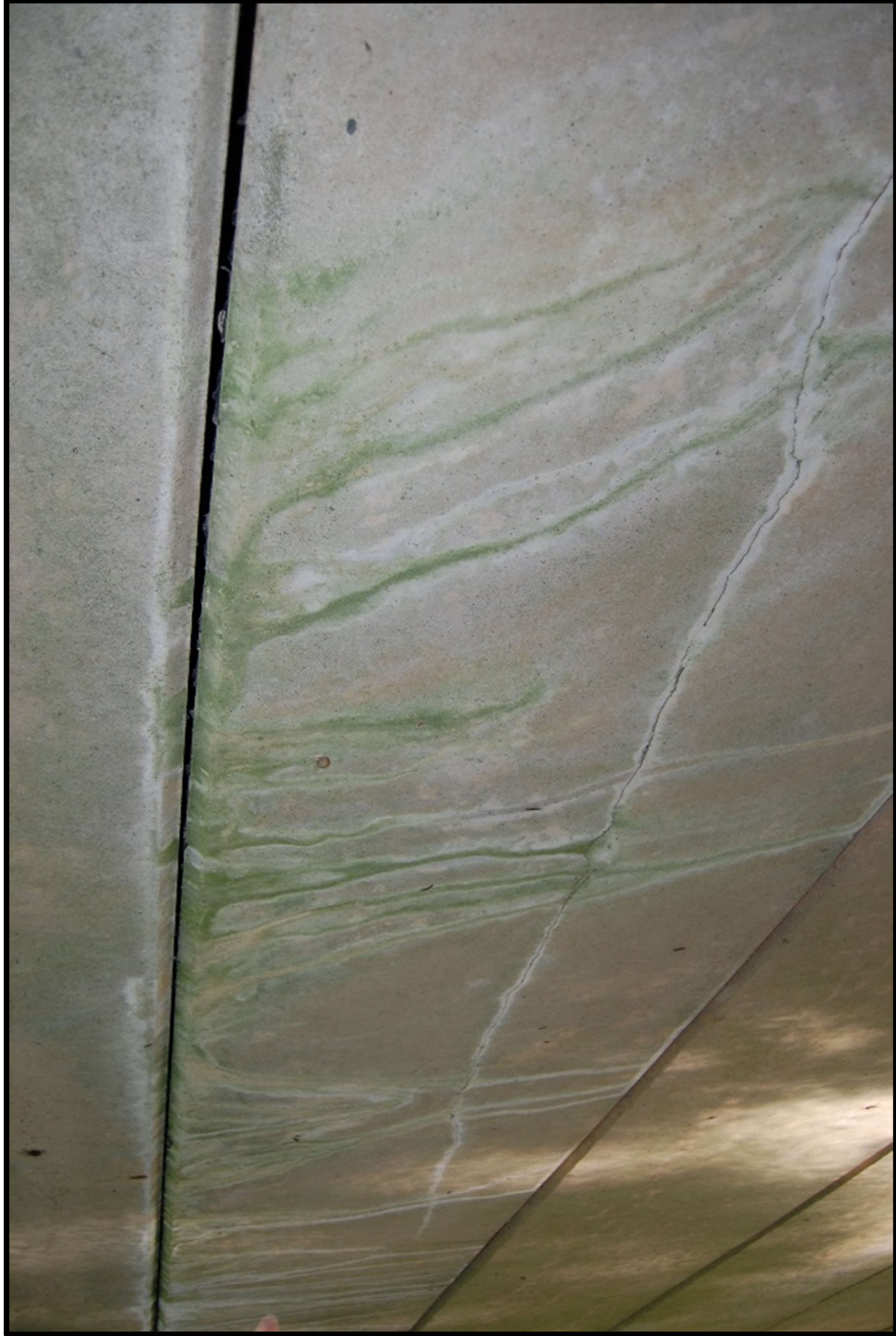
Figure 4.6 Longitudinal crack and staining at first interior beam.
