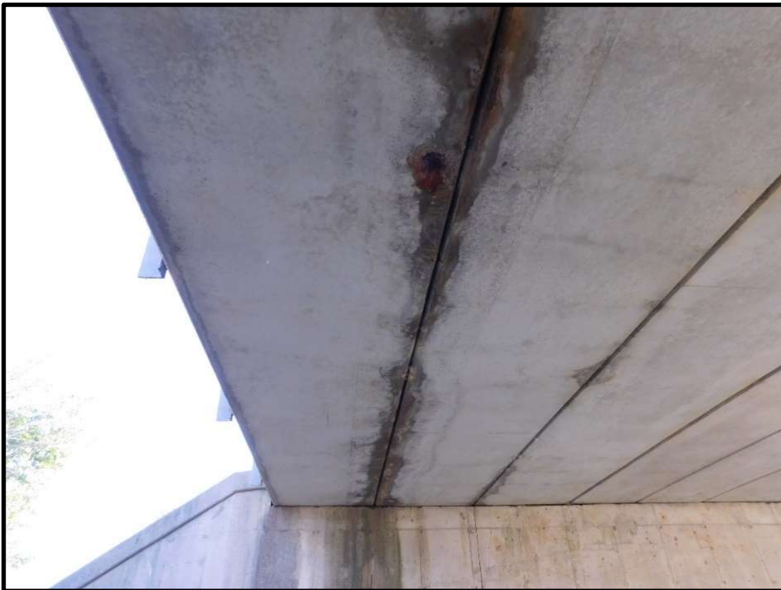
Figure 4.44 Leaking exterior joint (Beal-Taylor Ditch).
