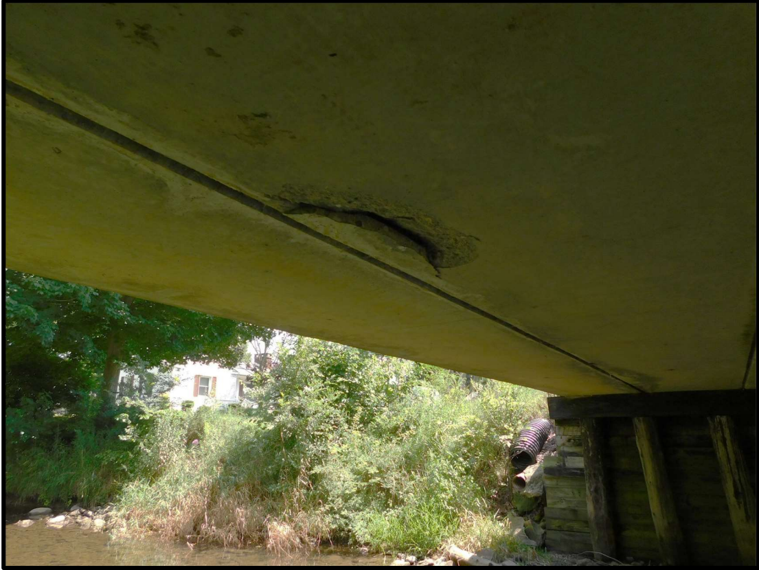
Figure 4.20 Spalling with exposed strand on Beam 7.
