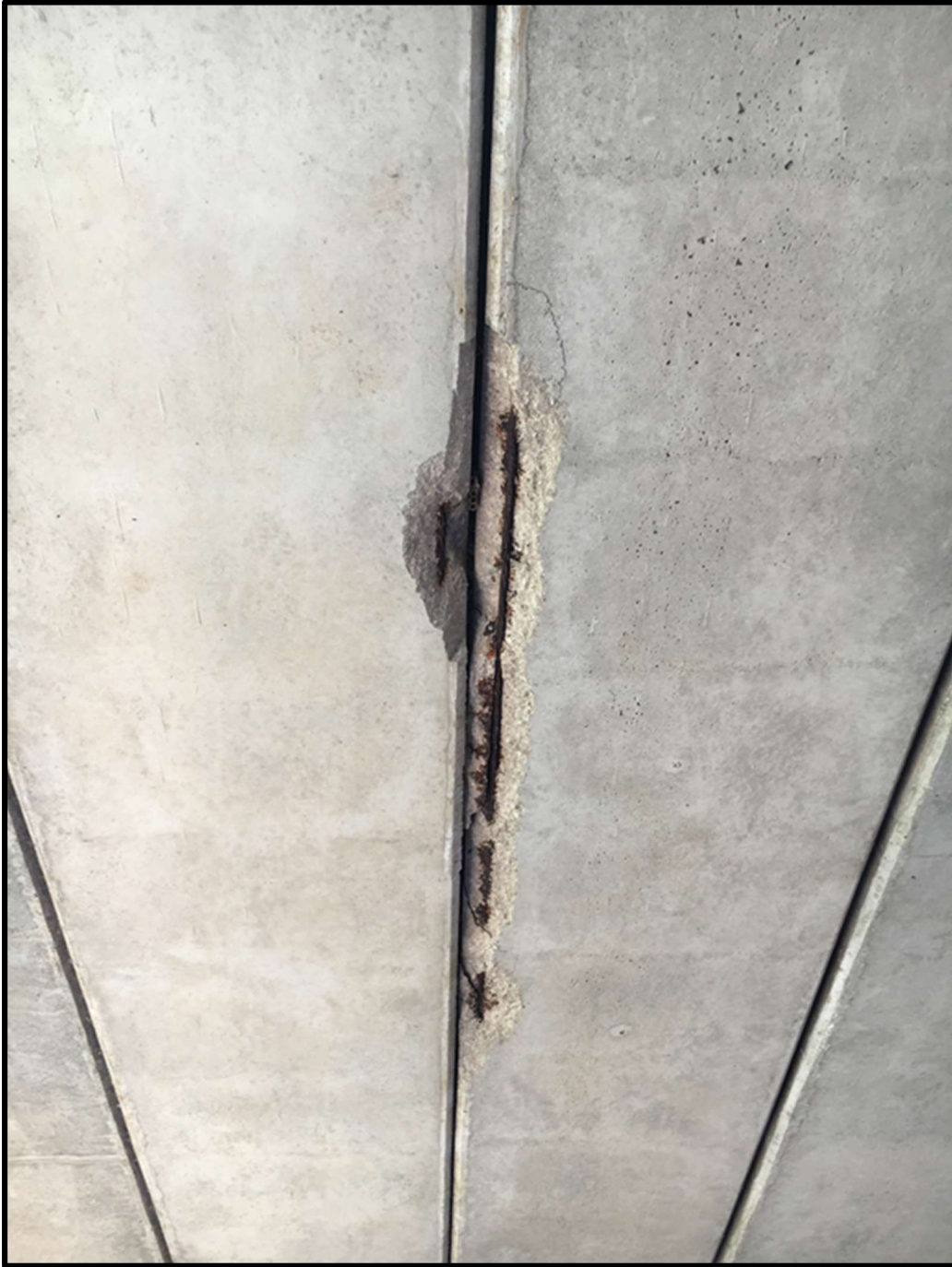
Figure 4.37 Spalling and exposed strand in the bottom corner of box beam (Clear Creek).
