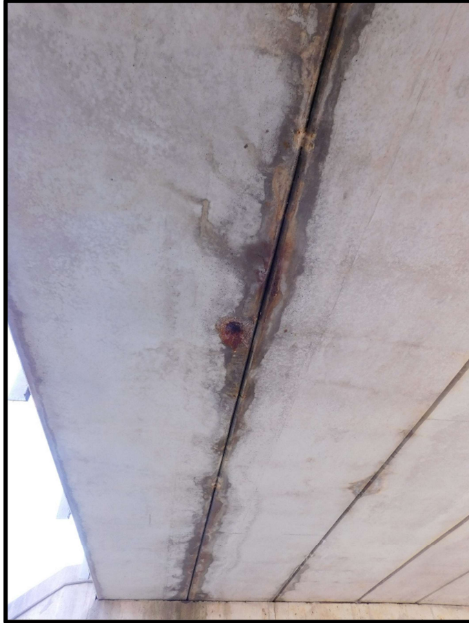
Figure 4.26 Efflorescence, spalling, and corrosion along bottom of exterior joint.
