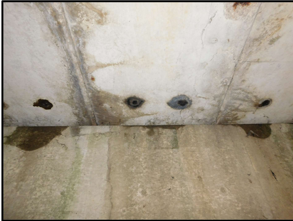
Figure 4.43 Black residue around drain holes (Main Street).
