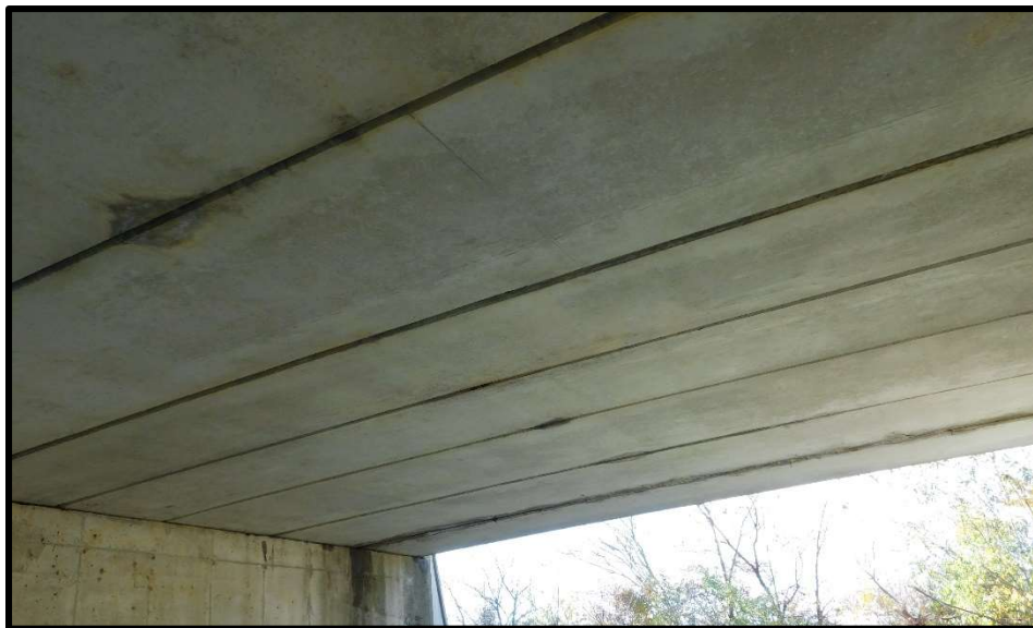
Figure 4.27 Efflorescence along bottom of interior joint.
