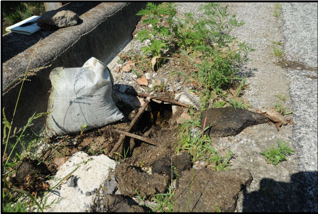
Figure 4.10 Hole in top flange of box beam.
