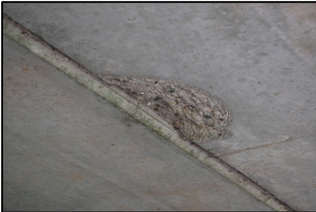
Figure 4.36 Spalling near longitudinal joint (Yellow Creek).
