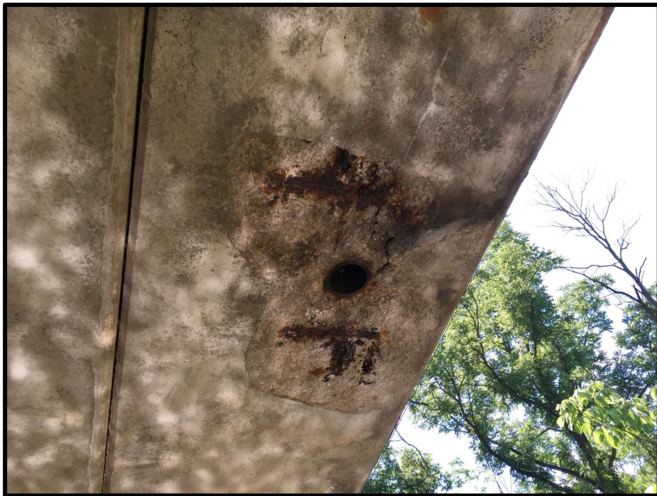
Figure 4.16 Corrosion and exposed stirrups around steel downpipe.
