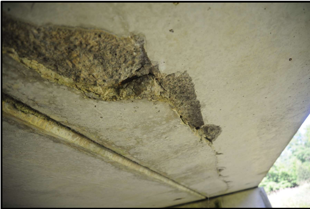
Figure 4.9 Exterior beam with spalling and exposed stirrups.
