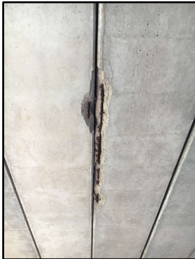
Figure 4.14 Region of spalling with two exposed strands.
