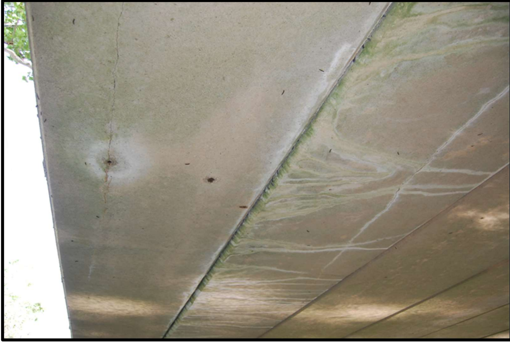
Figure 4.34 Water staining at the exterior longitudinal joint (Pond Creek).
