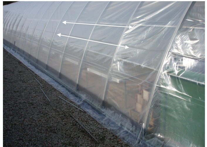
Figure 17. Positioning of polyethylene is simply done by aligning gusset creases with wall purlins.
