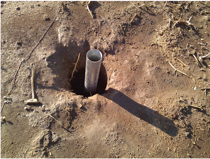
Figure 14. To create a pier foundation for the hoops, holes are drilled into the soil and filled with concrete around the ground posts.
