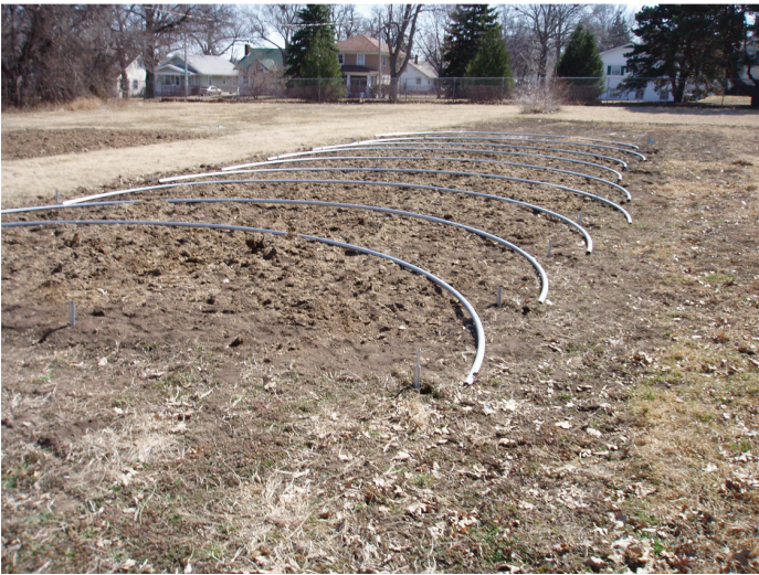
Figure 15. Assembled hoops located near ground posts ready to be tilted into position.
