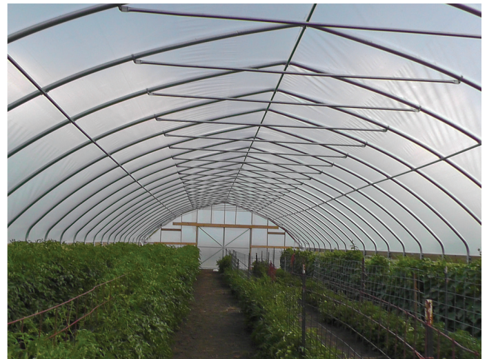
Figure 11. Cross bracing was installed in the peak of this high tunnel to stabilize the structure during high winds, heavy rains, and snowfall.
