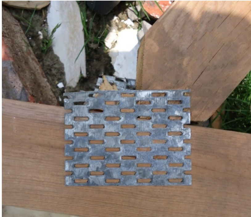
Figure 5.14, Example of connector with unequal overlap of the connector similarly observed in several locations. The gap between the wood members was within the range allowed at the time.
