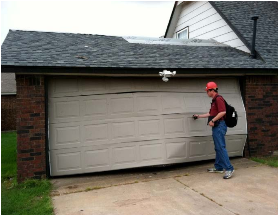
Figure 5.1, Partially collapsed light-gage metal garage door of house on tornado damage fringe.
