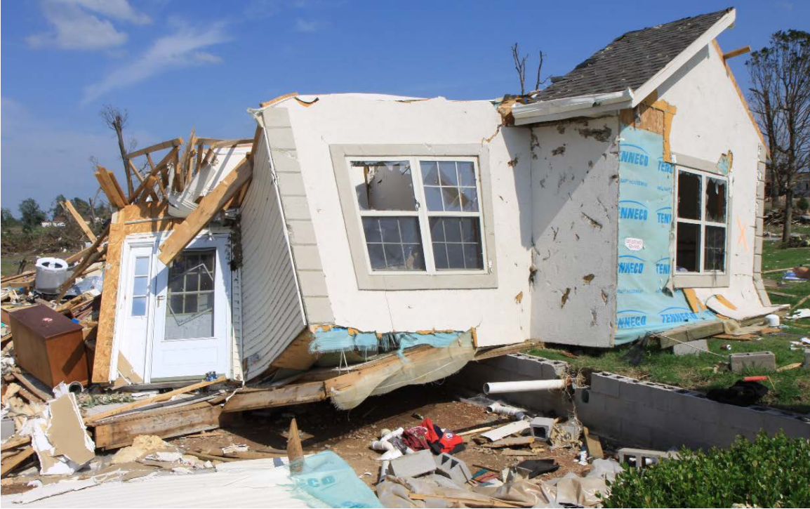
Figure 5.19, House shifted off of foundation in Joplin, MO after 2011 Tornado.
