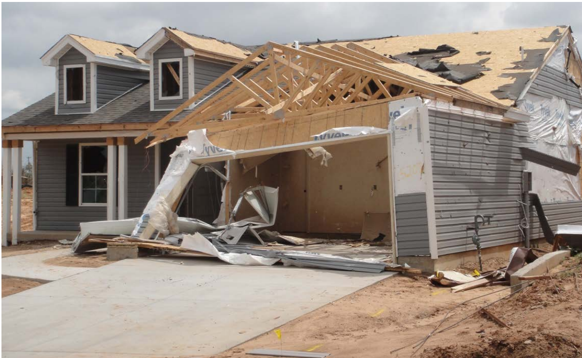
Figure 5.26, Stage 4 -- Garage Wall Framing Starts to Fail
