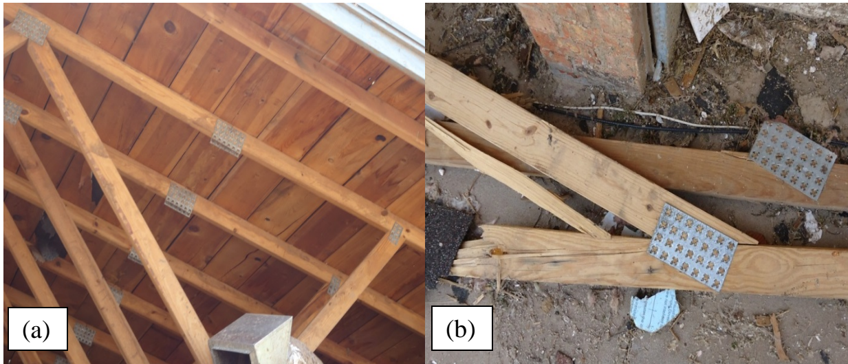
Figure 5.18, (a) Larger truss connector plates than for 808 S. Silver Leaf and (b) example of failure within the truss members.
