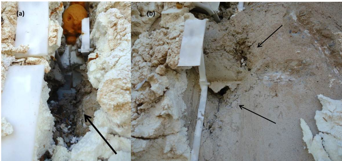
Figure 4.11, Inadequate concrete pour indicated by; (a) a large area of poorly consolidated concrete below missile perforation and (b) a large void in the concrete in the thinned area of the waffle grid and in the vicinity of a plastic clip.
