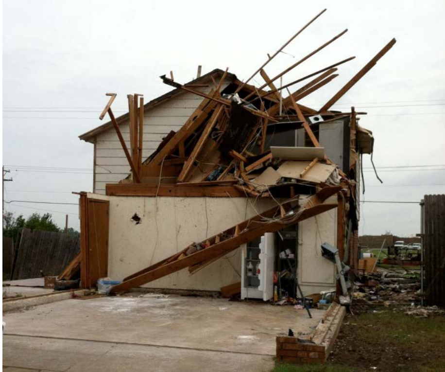
Figure 5.3, Missing garage on house with “protruding” garage.
