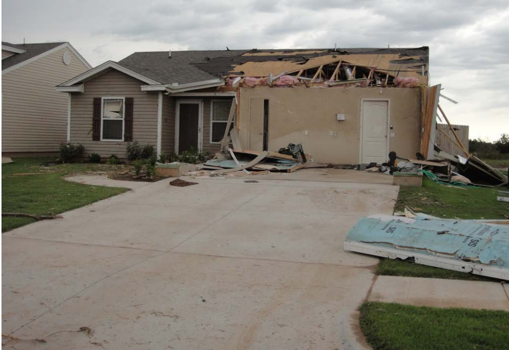
Figure 5.27, Stage 5 -- Garage Completely Destroyed; Main Roof Begins Peeling Off; Attic is now partially Enclosed
