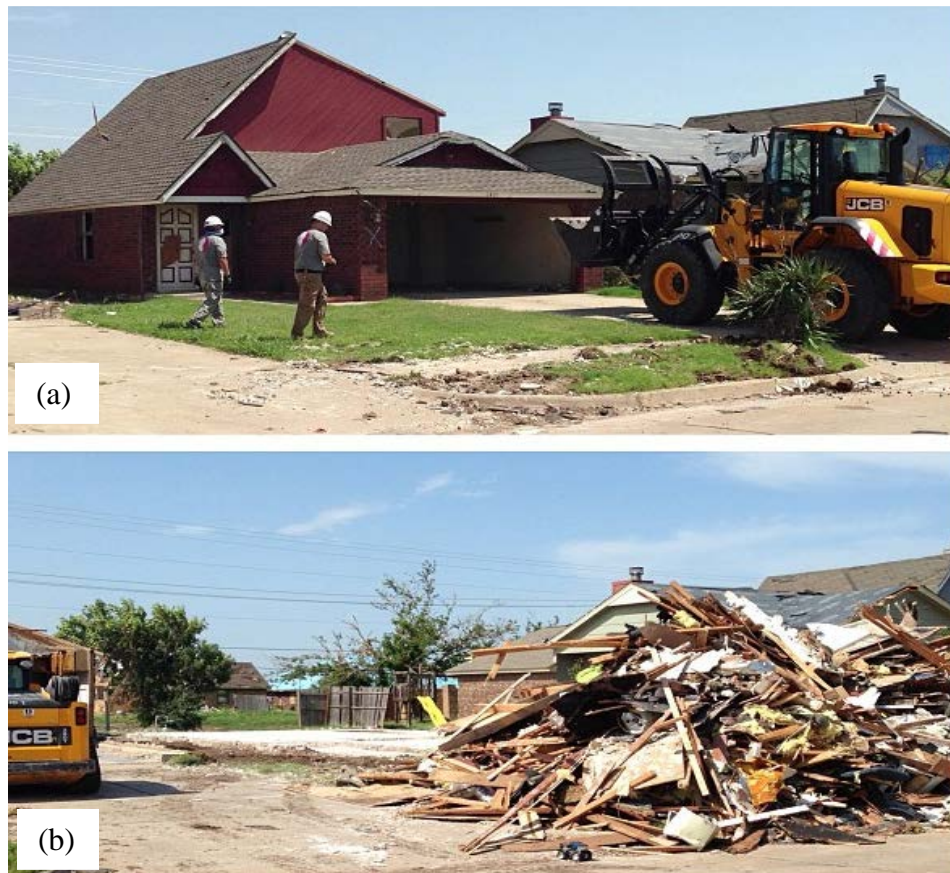
Figure 3.3, Comparison of damaged home (a) pre- and (b) post-demolition
