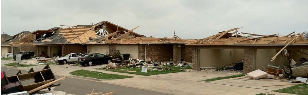
Figure 5.8, Progression of roof damage to “high profile” ridge beam/rafter roofs.
