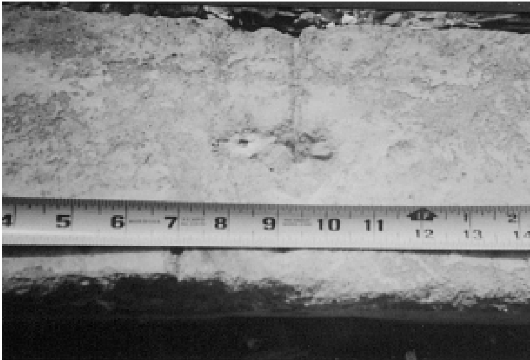
Figure 5.22, Scrape mark in the surface of concrete slab foundation indicating where the wall bottom plate along with the tapered cut nail connection were moved laterally (Marshall, 2002).
