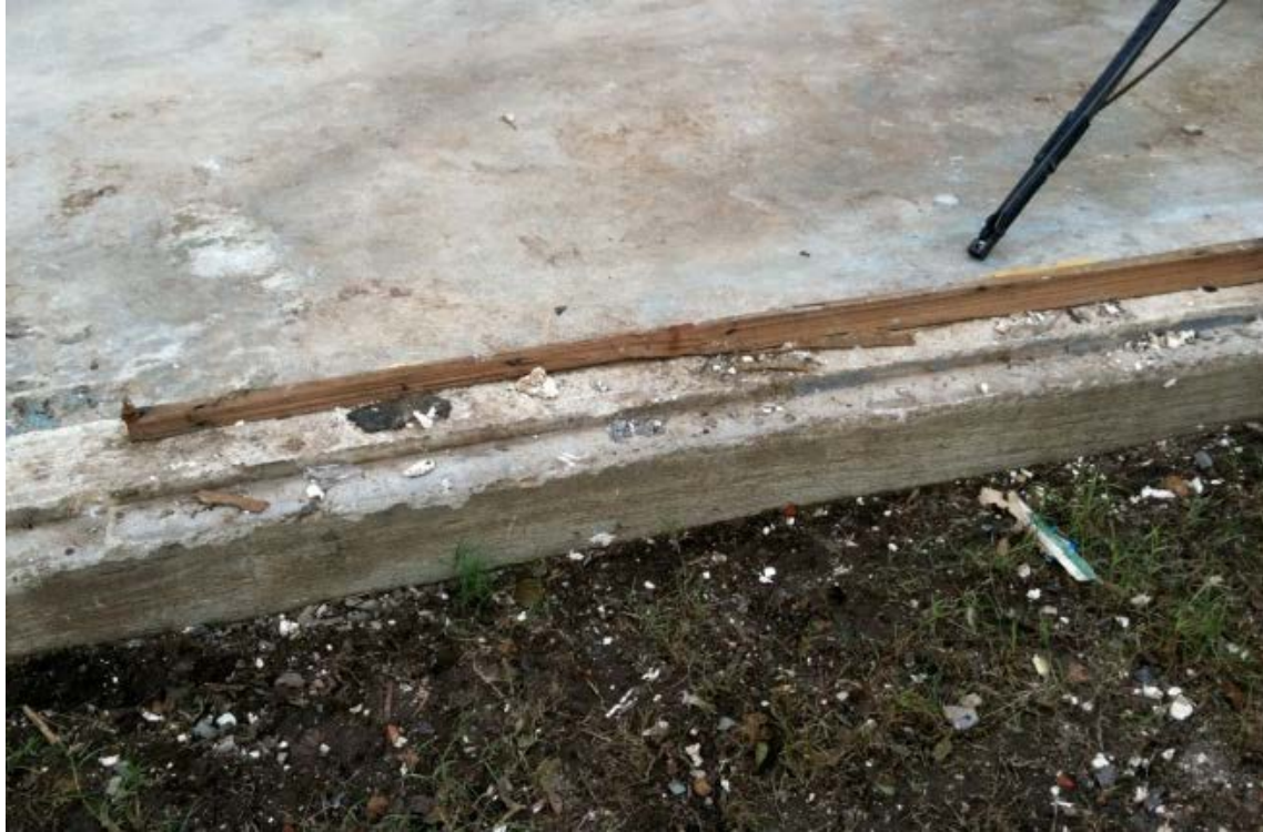
Figure 5.4, Failed sill plate with anchor bolt still attached.
