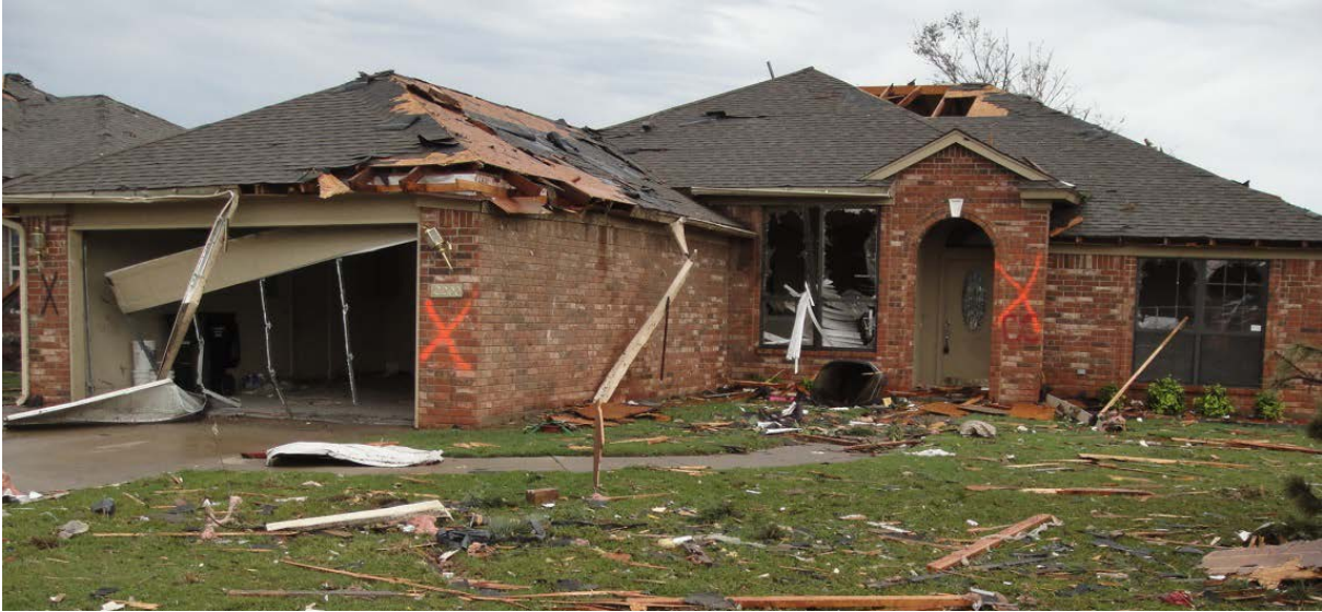
Figure 5.25, Stage 3 -- Home Becomes Partially Enclosed Structure; Roof Begins Peeling Off
