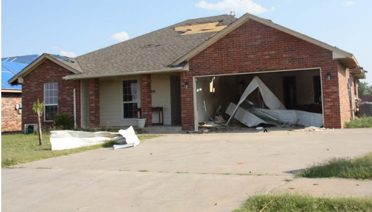
Figure 5.24, Stage 2 -- Garage Door Completely Destroyed
