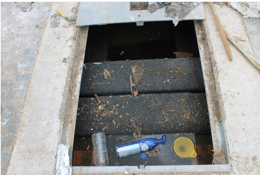
Figure 4.5, Flooded storm shelter from severed water lines and rain. Floating debris indicates that water has reached the top of the storm shelter.
