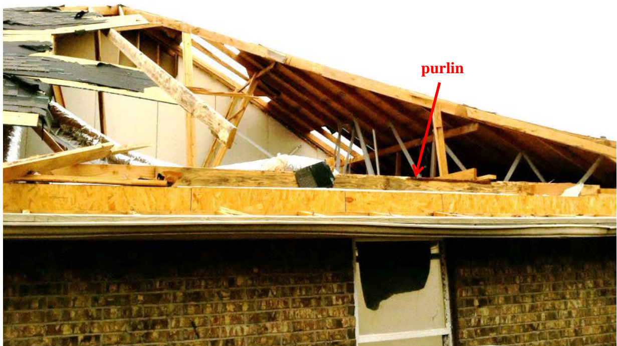
Figure 5.7, Long unsupported spans of rafters on typical “high profile” roof. Lateral support to bottom of rafters indicated by red arrow.
