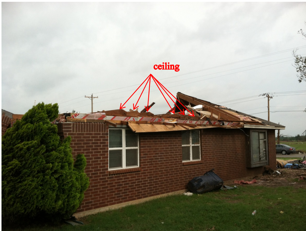
Figure 5.6, Missing roof but intact ceiling joists.
