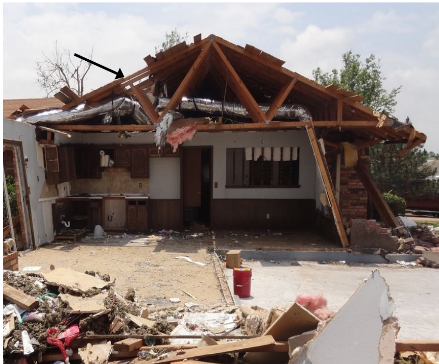
Figure 5.12, Intact roof truss with plate failure location indicated.
