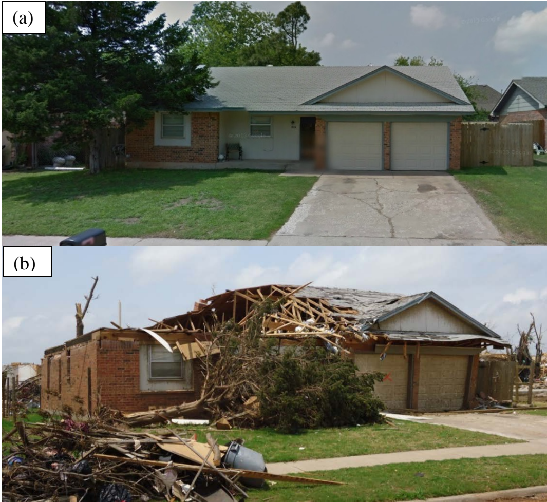
Figure 5.15, 805 S. Silver Leaf Drive (a) before (Google Maps, 2013) and (b) after the tornado. The Degree of Damage (DOD) on the EF scale was 6 based on the removed roof structure and most walls remaining intact, which suggests wind speeds between 104 and 142 mph with an expected speed of 122 mph.
