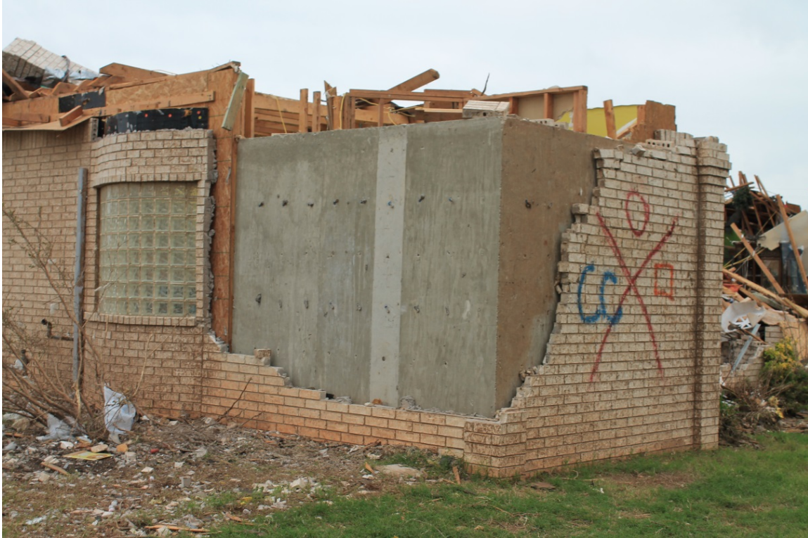
Figure 4.6, FEMA designed CMU safe room found near Riverside Drive in eastern Moore.
