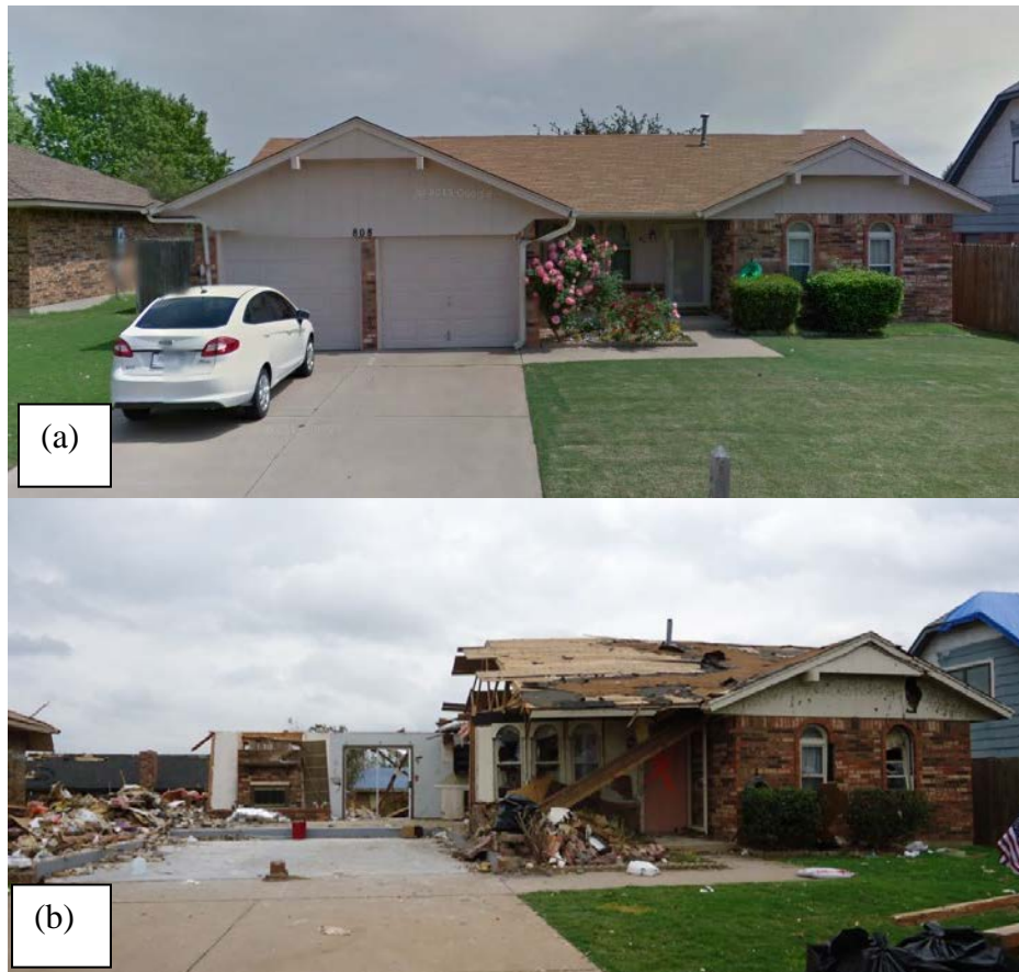
Figure 5.10, 808 S. Silver Leaf Drive (a) before (Google Maps, 2013) and (b) after the tornado. The Degree of Damage (DOD) on the EF scale was 6 based on the removed roof structure and most walls remaining intact, which suggests wind speeds between 104 and 142 mph with an expected speed of 122 mph. The collapsed walls indicated a DOD nearer to 7 and wind speeds toward the high end of this range.
