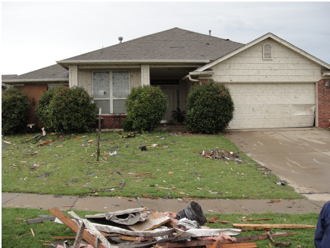
Figure 5.23, Stage 1 -- Wind Pressure Initiates Failure of the Garage Door
