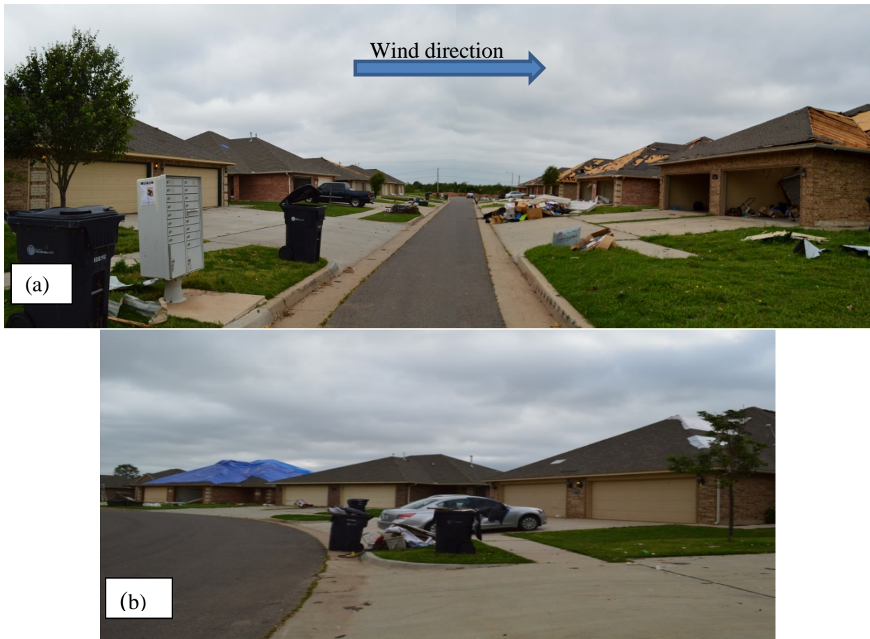
Figure 7.2, Different garage door damage levels (a) on both sides of SW 151st Street and (b) when house directions change.
