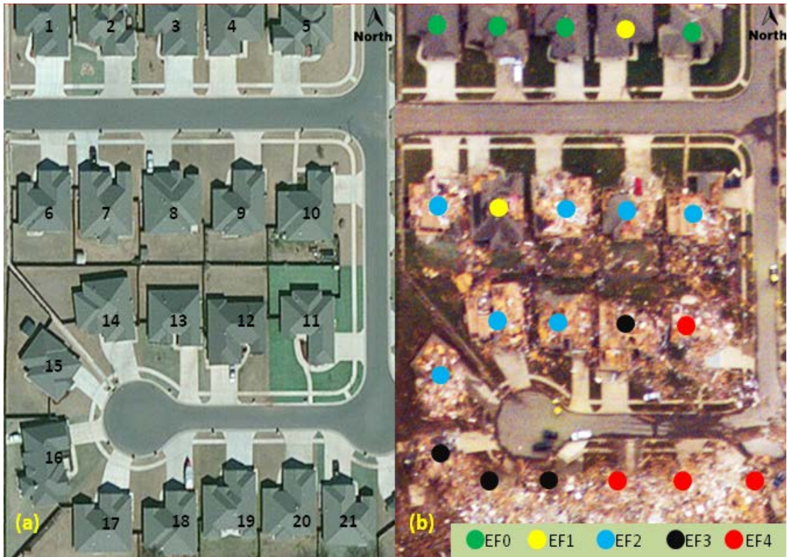
Figure 2.9, Aerial images and EF rates of the area #1: (a) pre-tornado image and building IDs; (b) post-tornado image and EF rates.
