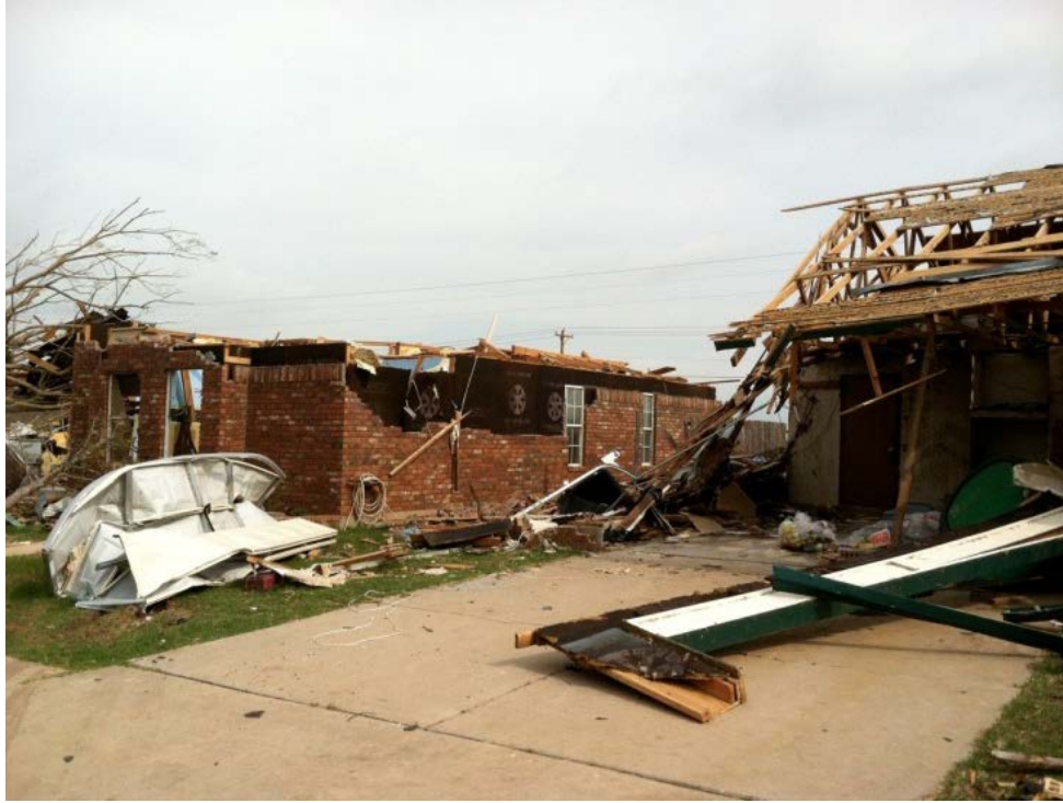
Figure 5.5, Missing rafter/ridge beam roof on house to left of house with largely intact prefab truss roof.
