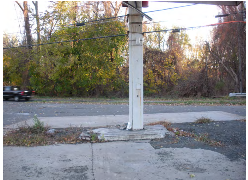
Figure 3.13 shows exposed soil not native to the area
