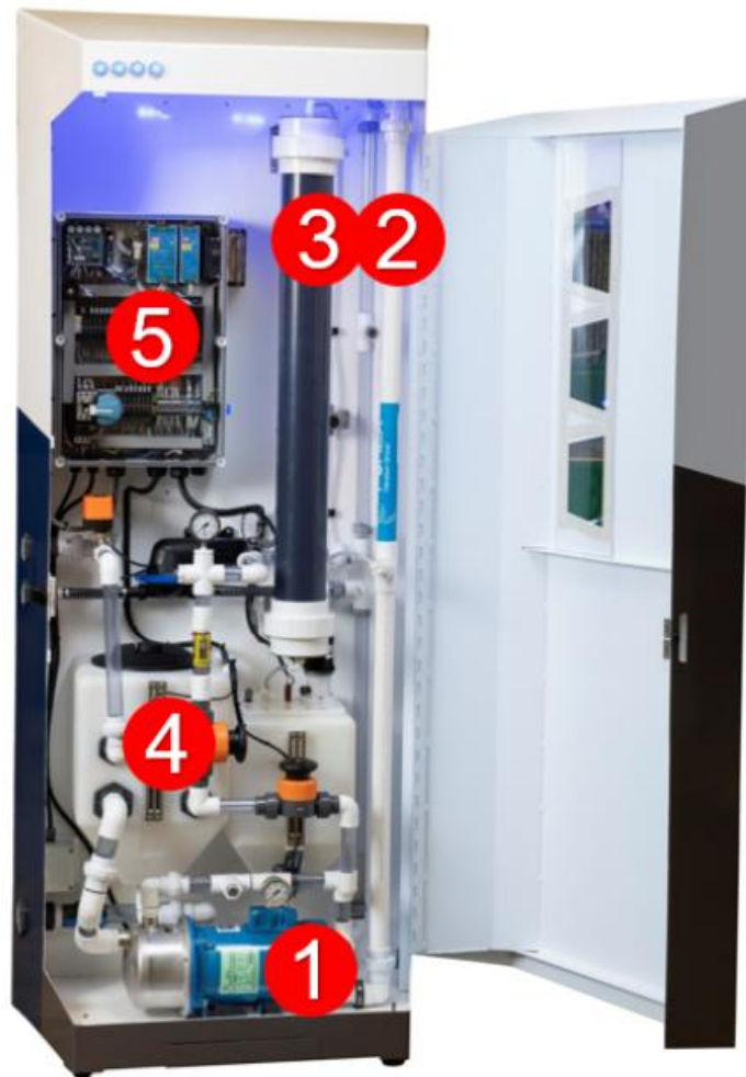
Figure 1. The following elements are highlighted in the image of the Duke Center for WaSH-AID liquid waste treatment system: 1. Ultrafiltration pump 2. Ultrafiltration membrane 3. GAC column 4. Electrochemical cell 5. Controls system
