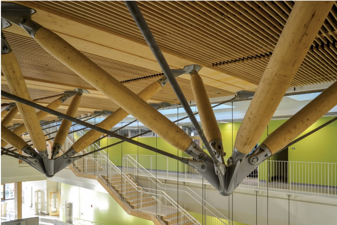
Figure 5. Connection details of zipper trusses at the John W. Olver Design Building (Leers Weinzapfel Associates; Amherst, MA, USA; 2017) at University of Massachusetts Amherst. (Miller 2017)
