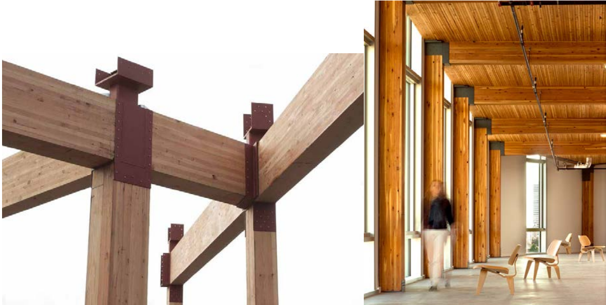
Figure 1. Steel connections between glulam elements at the Bullitt Center (Miller Hull Partnership; Seattle, WA, USA; 2013). Left: during construction (Court 2012), photo by John Stamets; right: interior after completion (Schuchart n.d.).
