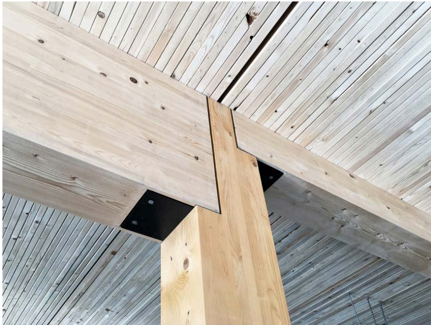
Figure 3. Structural connection detail at T3 (Michael Green Architecture and DLR Group; Minneapolis, MN, USA; 2016). (Brownell 2016)
