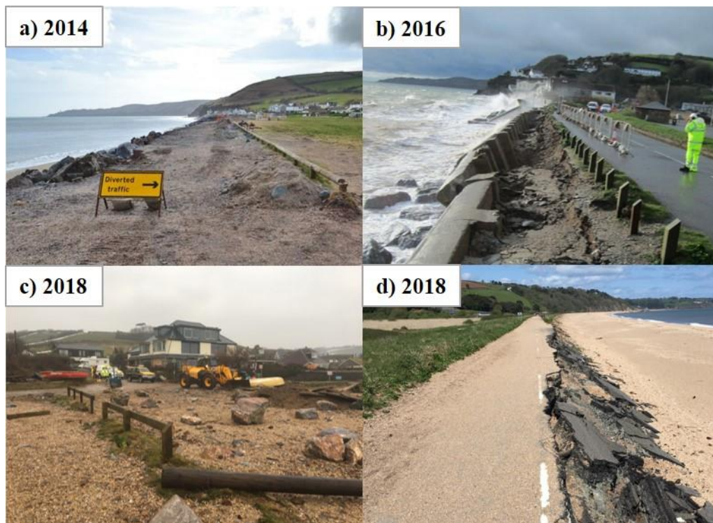
Figure 1.10. Contemporary storm damage issues in Start Bay a) Road destruction at Beesands following southerly waves brought in by Storm Petra, February 2014, b) undermining and collapse of sea wall at Torcross, Slapton Sands following sustained southerly incident waves and lowest recorded beach levels in February 2016, c) evacuation of residents following high tide impact of Storm Emma, March 2018, d) the second collapse of the A379 road atop the Slapton Sands barrier ridge following Storm Emma, March 2018.
