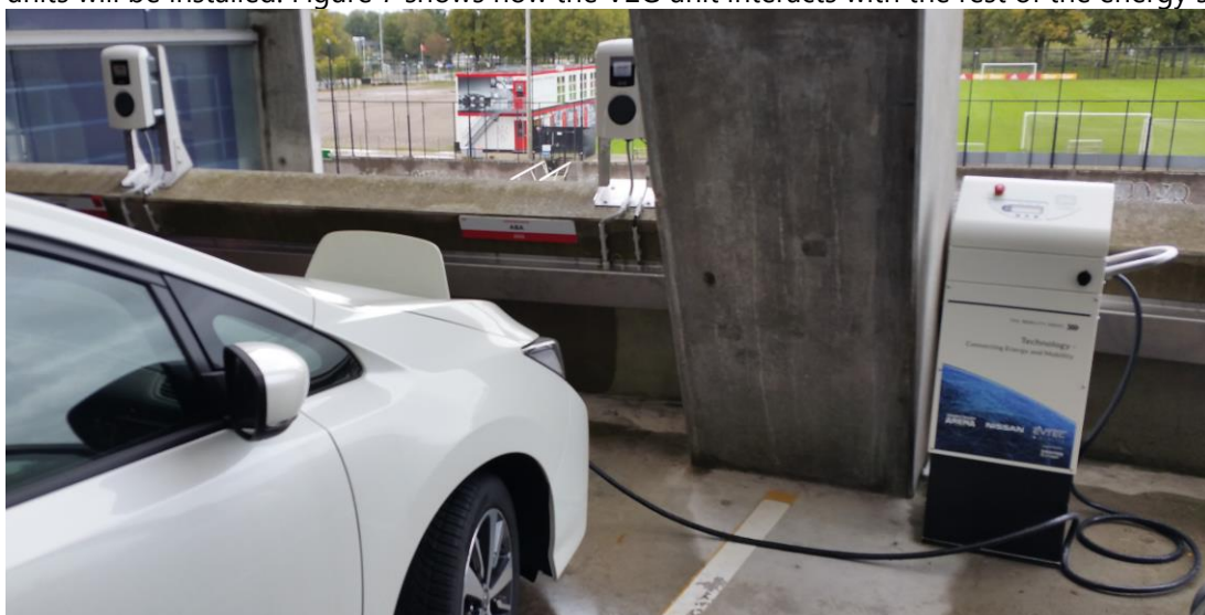
Figure 6: Two of the EV chargers (on the left) and the V2G unit (on the right).
