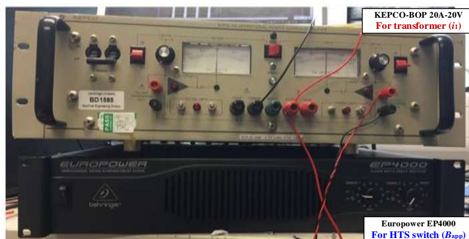
Fig. 4.11. Two power supplies used to power the transformer and HTS power switch: (a) KEPCO-BOP 400W 20A-20V bipolar operational power supply, and (b) Europower EP4000 power supply.
