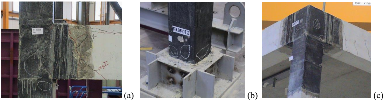
Fig. 5 - Damage after the test at PGA=0.5g on the CFRP strengthened frame: (a) beam end at 1 st storey, (b) bottom of column 1 st storey, (c) 2 nd storey joint
