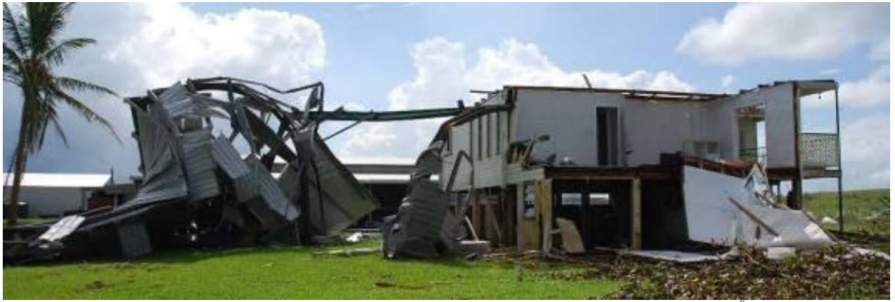
Figure 8: Effect of large scale debris on house. Courtesy of Cyclone Testing Station, James Cook University 9
