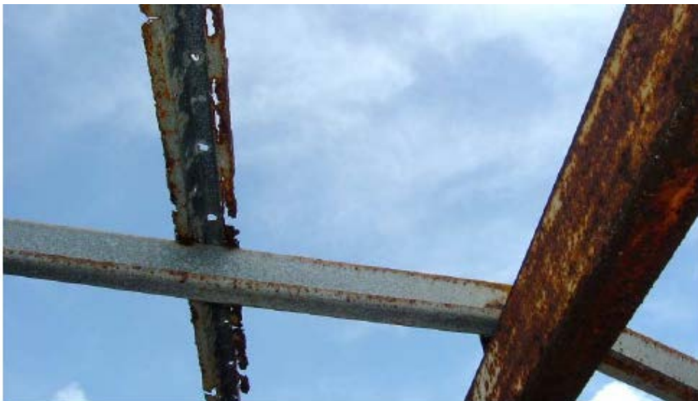
Figure 6: Detail of corrosion of top hat batten, courtesy of Cyclone Testing Station, James Cook University 14
