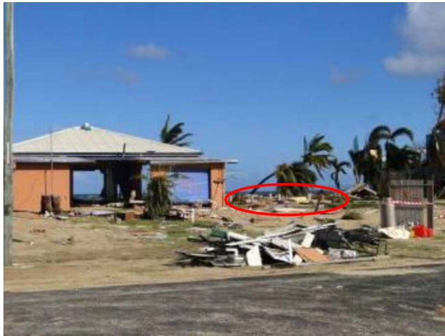
Figure 4: Houses at Tully Heads. Red ring marks position of house demolished by storm tide. Courtesy of Cyclone Testing Station, James Cook University 9
