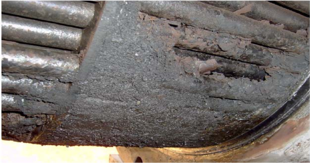
Figure 2-6. MEG regeneration unit tube bundle fouled by \text{FeCO}_3 (Latta [10])
