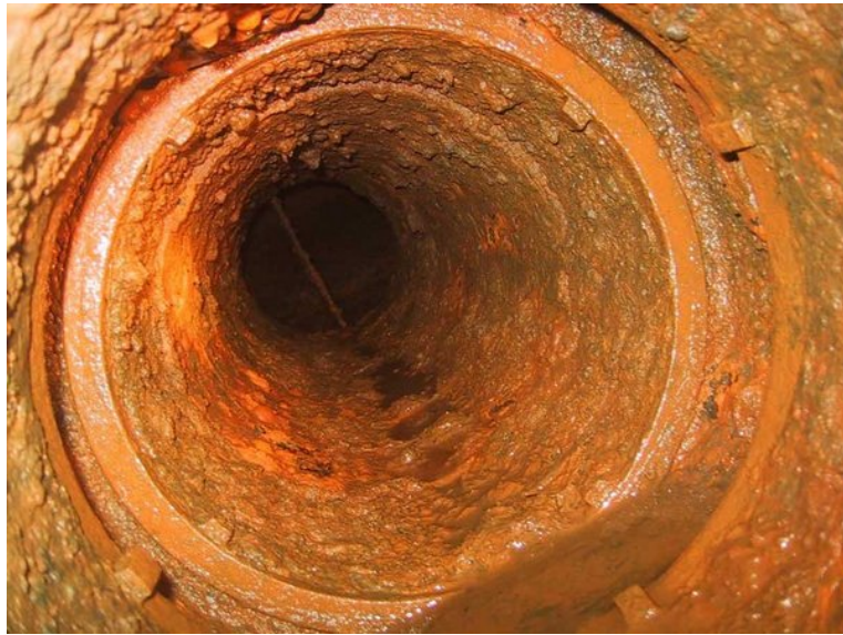
Figure 2-8. Internal corrosion of a natural gas pipeline (Popoola [98])
