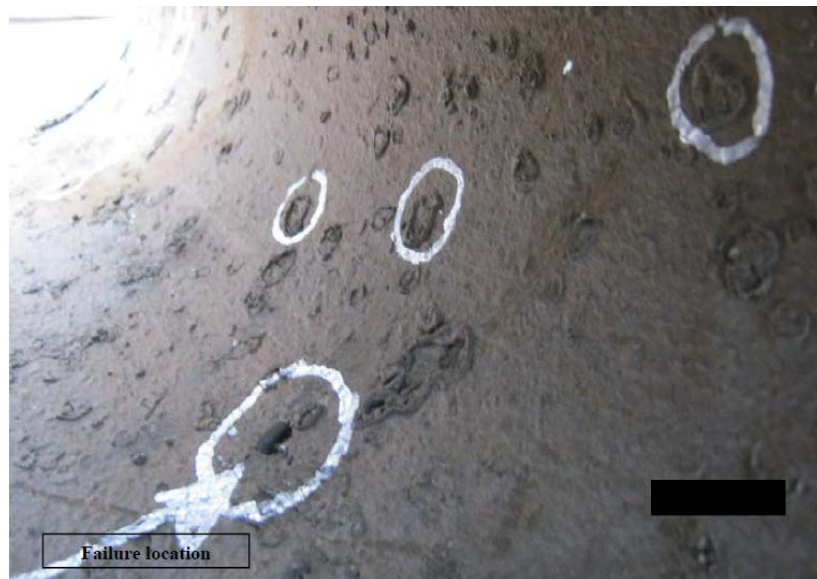
Figure 2-9. Pitting failure of a natural gas pipeline (Mansoori [82])
