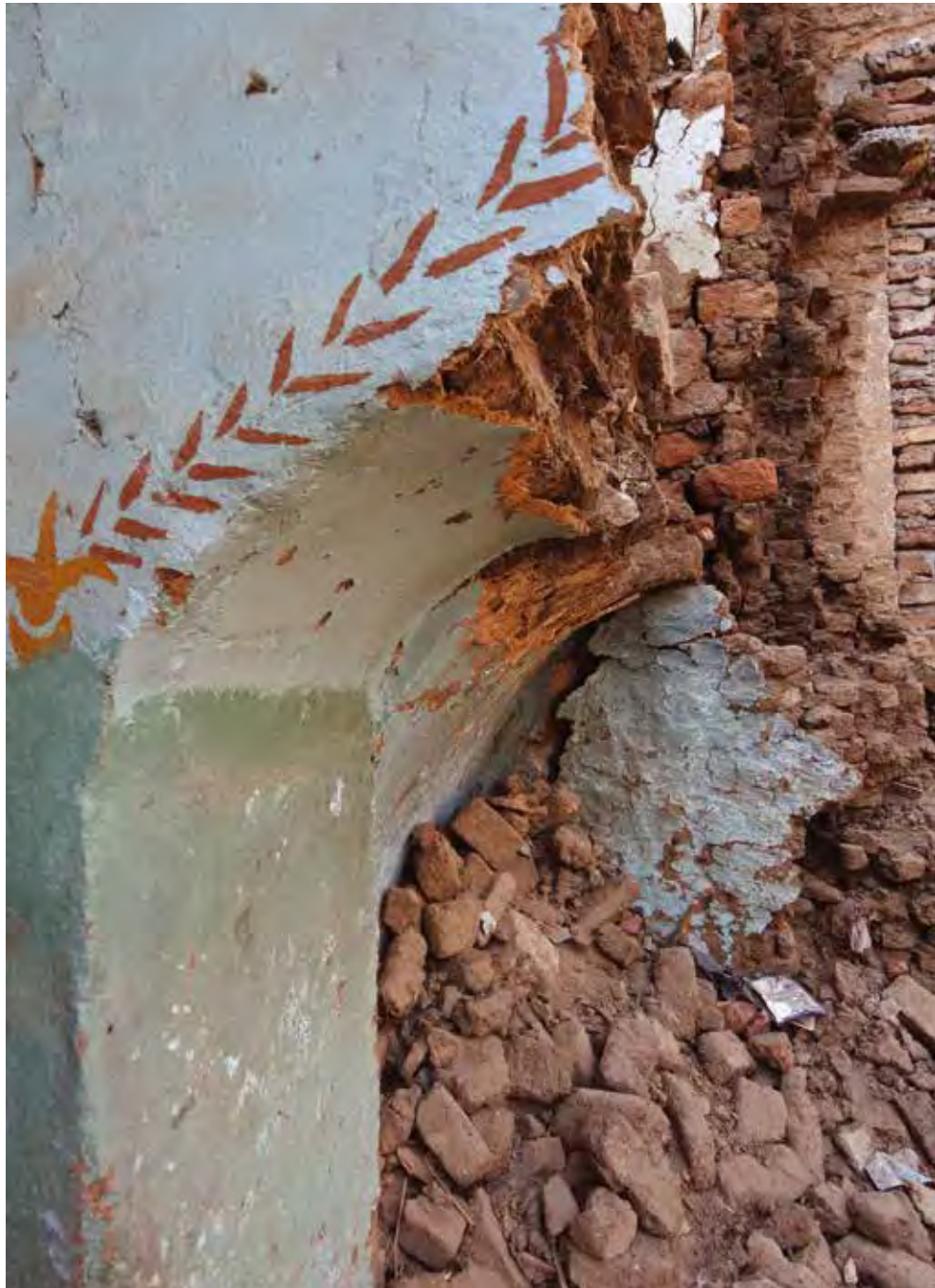
Decaying mudbrick wall in New Gourna. Photo: Zs. Vasáros, 2018.
