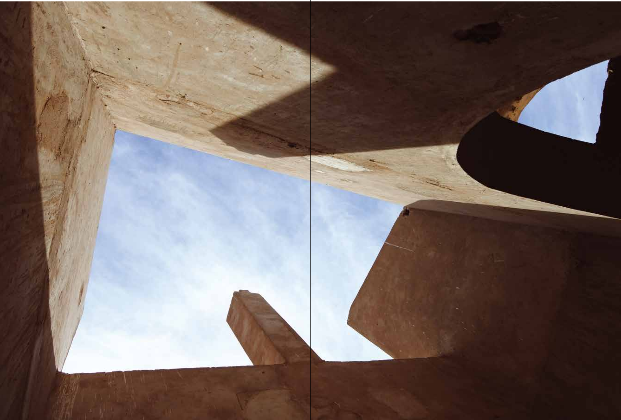
Ventilation shaft in the Sadat Rest House, Gerf Hussein. Photo: Zs. Vasáros, 2017.
