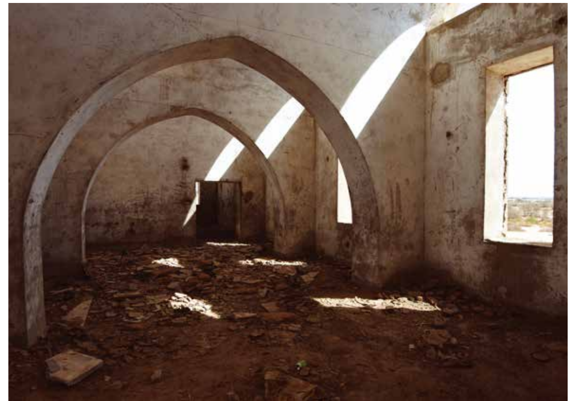
The destroyed interior of the Rest House. Photo: Zs. Vasáros, 2017.
