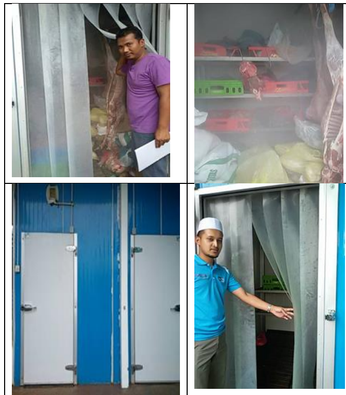
Images 4.4: Freezer, Chiller, and Refrigerator
