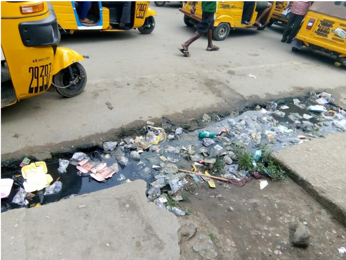
Figure 5: A Refuse-blocked gutter near Aba Main Park
