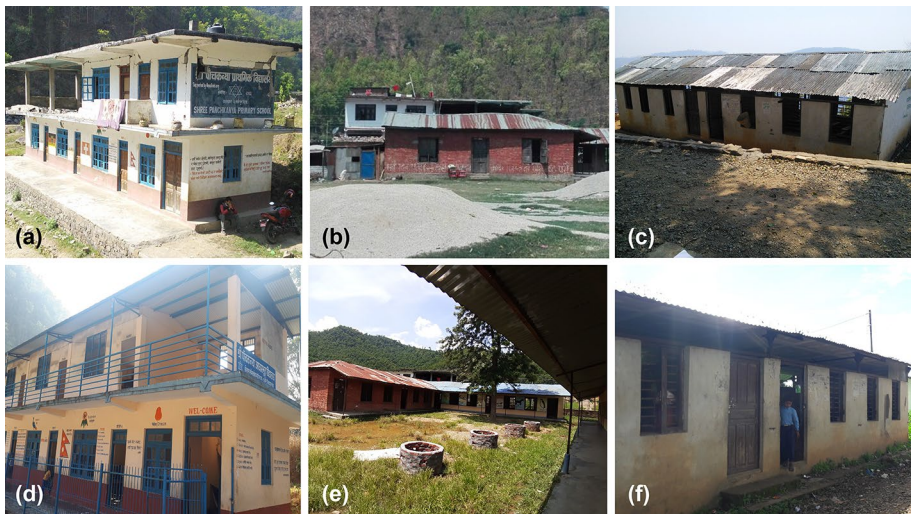
Fig. 2 Shree Pachkanya Primary School (EMIS230350008, Building A)—RC frame typology: a SIDA, d SAFER. It can be observed that the earthquake damage detected in 2016 by SIDA surveyors has been subsequently repaired as shown in the SAFER database. Shree Narayan Devi Higher Secondary School (EMIS280330001, Building B)—Masonry typology: b SIDA, e SAFER. Seti Devi Higher Secondary School (EMIS230770009, Building D)—steel frame typology: c SIDA, f SAFER
