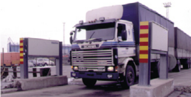
Figure 9. Automatic portal radiation monitor controlling cargo traffic at the Port of Helsinki.
