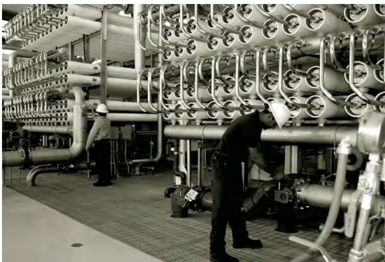
FIGURE 26.8 El Paso water utilities desalination plant. (Courtesy of El Paso Water Utilities.)
