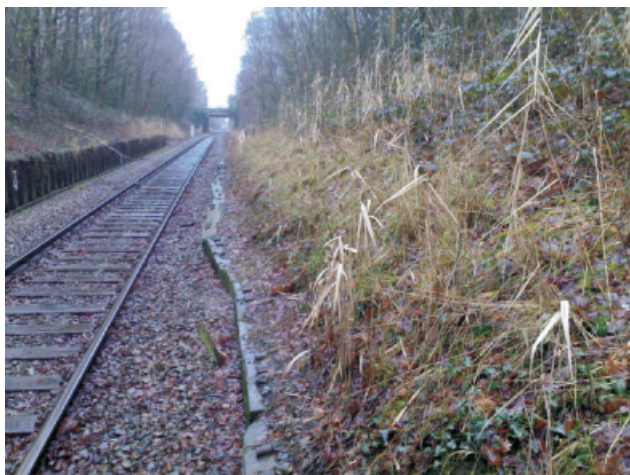
Figure 4. The toe of the slope, showing the distorted concrete cable trough and toe bulging
