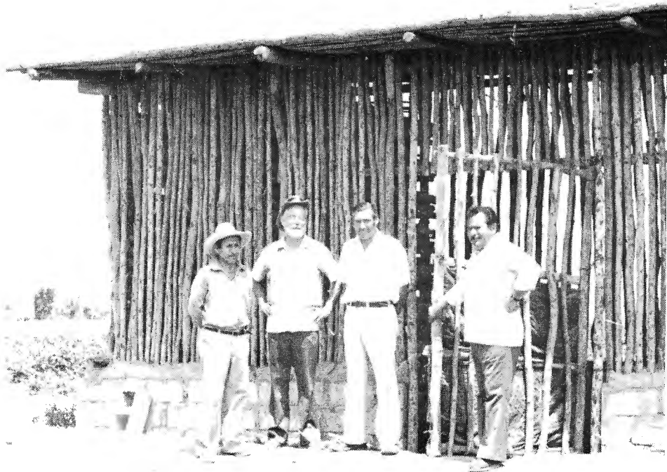
Figure VIII-1. Demonstration diffused light seed store constructed on a potato producing cooperative in the coastal area of Peru as part of a INIA/CIP collaborative storage contract. As a result of this demonstration the same cooperative constructed a similar store with a capacity of 80 to 110 metric tons of seed tubers.
