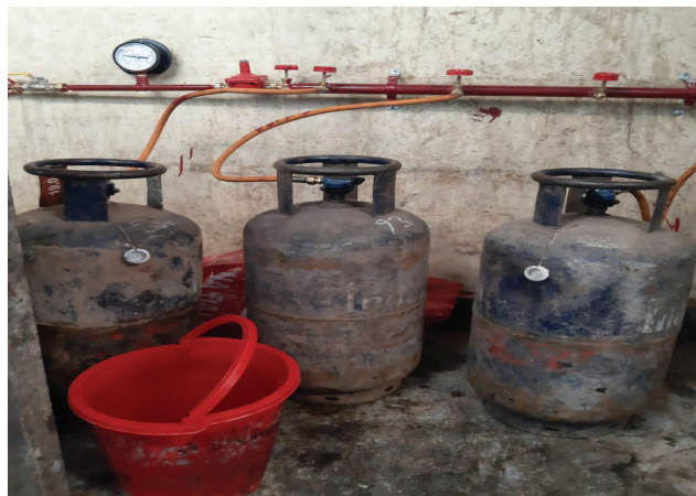
Cylinders are placed outside the preparation unit and connected through a common gas duct to the burners
