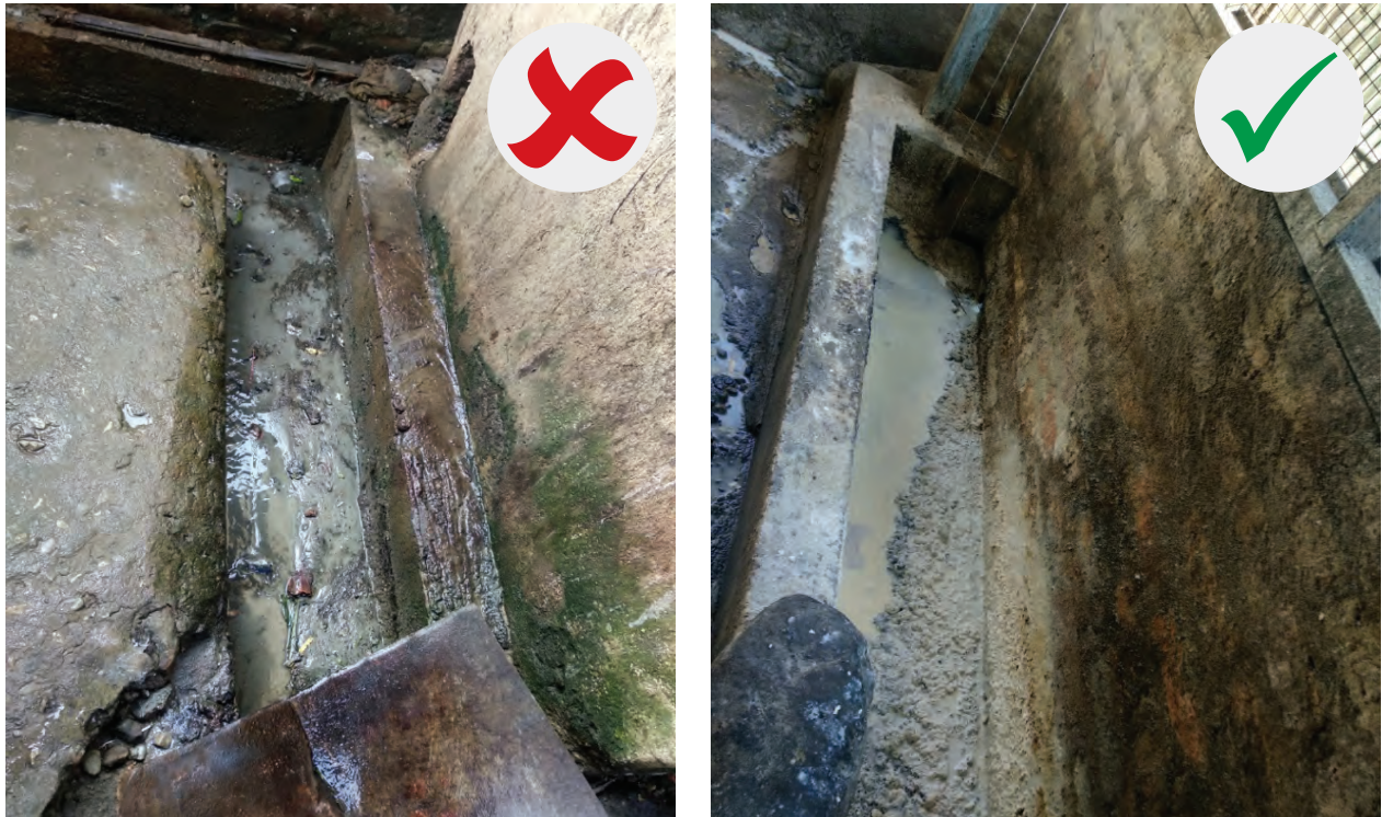
Common and improper drainage system of sweet making units in Assam
