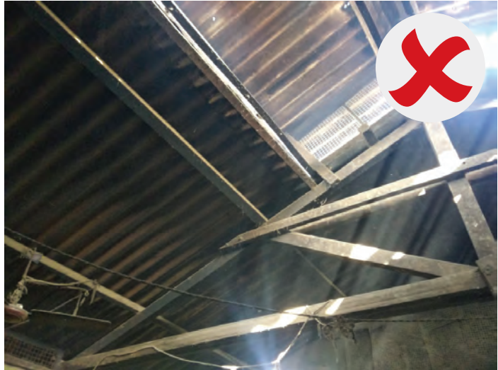
Ceiling without any cover with chance of falling particle/dust on finished products/raw materials
