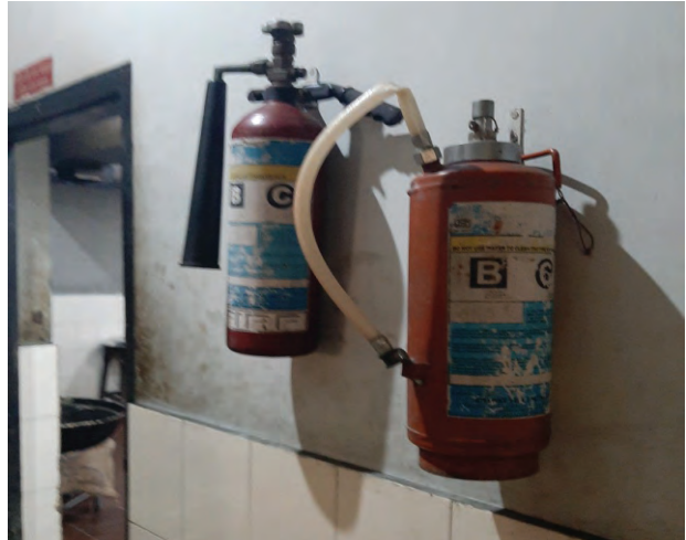
Placing of fire extinguishers at a handy place like in the entrance
