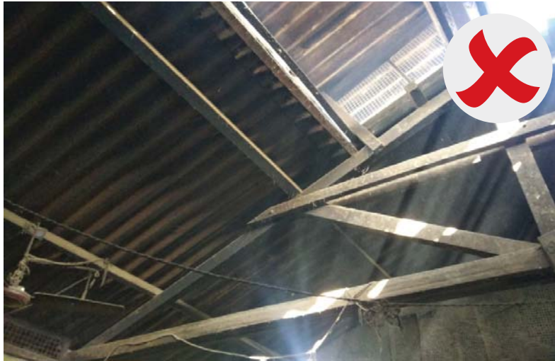
Ceiling with chance of falling particle/dust on finished products/raw materials
