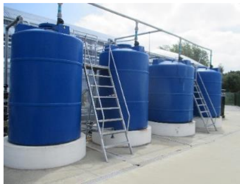
Figure 14 - Tanks for water storage and treatment at UEL.
