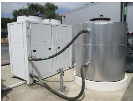
Figure 18 – Chiller in thermoregulation system.
