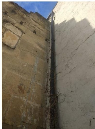
Figure 19: Pipe running along the intersection
