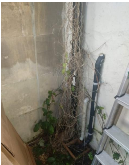
Figure 18: Pipes in the intersection of the walls is part of the boundary constraints
