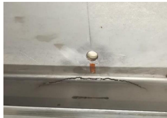
Figure 31 - Representative fatigue cracks (example).
