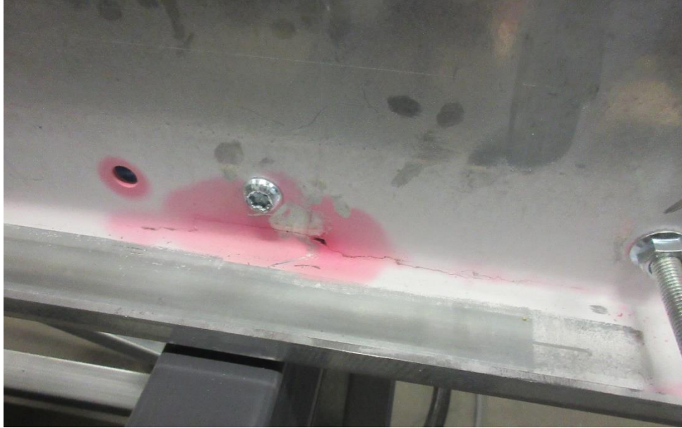
Figure 2 - Observed cracking due to material fatigue in a cold-formed steel rail.
