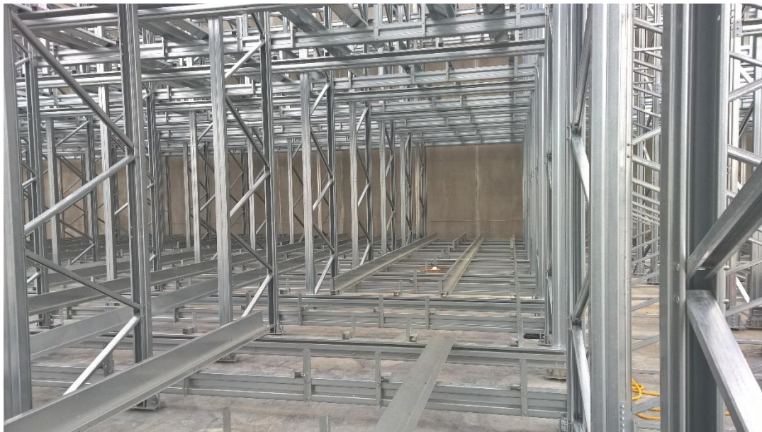
Figure 1 - Rack structure prepared for automatic pallet-carrying shuttles.
