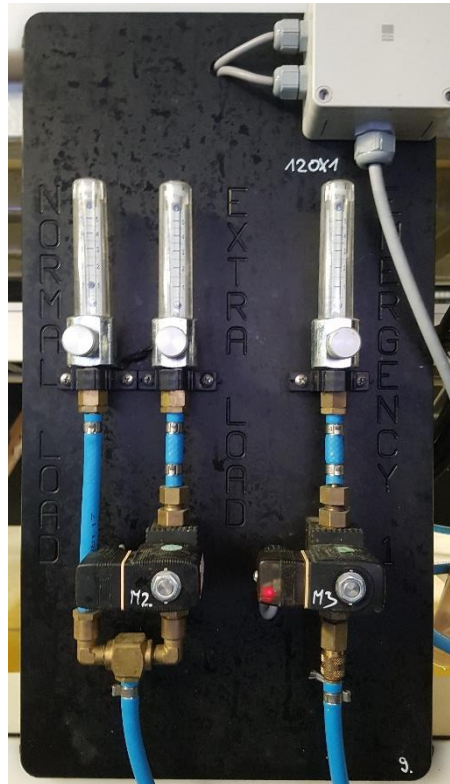
FIGURE 10 - OXYGENATION CONTROL PANEL AT BIGH
