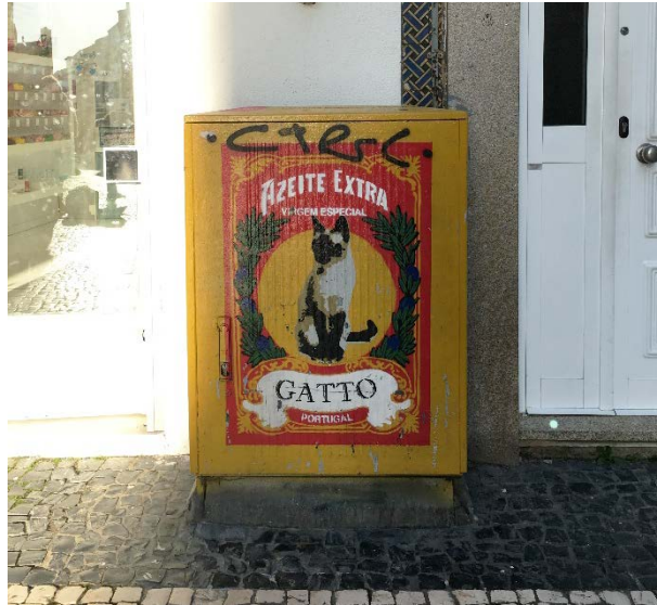
Image 32 – “Street Art Porto - Caixas EDP”: This is the result of the creativity of the artists challenged by Oporto’s Municipal chamber to painting the electrical distribution boxes that exist on the streets. This box is one of the many existing in Rua das Flores, a street highly frequented by tourists, which can be considered as strategic placement.
