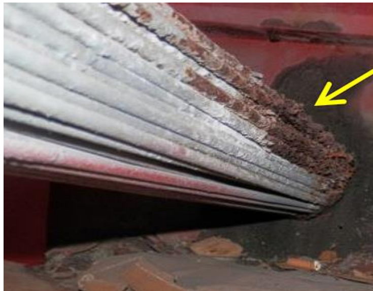
Figure 38 - Corrosion identify on the Edgar Cardoso Bridge [22]
