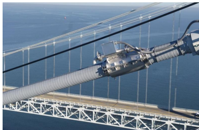
Figure 19 – Dehumidification system applied on the Bay Bridge, United States.
