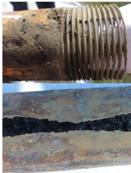
Figure 16 – (Top) corroded rising main thread; (Bottom) perforated rising main.
