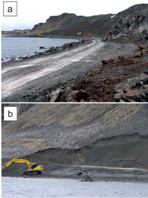
Figure 4 (a) Access road to Quarry No. 3, Fildes Peninsula, King George Island (Photo: H.-U. Peter); and (b) extraction of material within part of Quarry No. 3 (Photo: H.-U. Peter).
